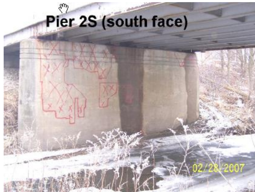
Figure 6-2: Shows after sounding, delaminations are marked on Pier wall
