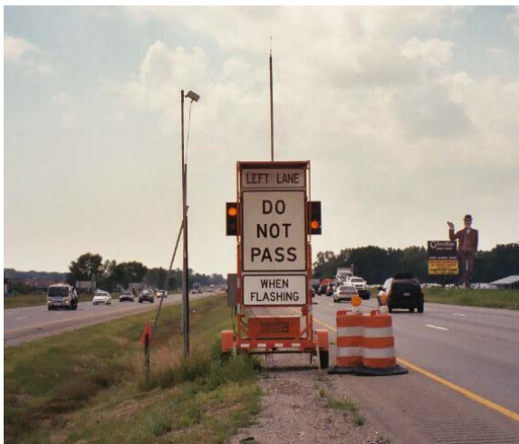
Photograph 6. Modified Set Up of the Sign Trailer and Sensor in a Depressed Median (2003 Construction Season)
