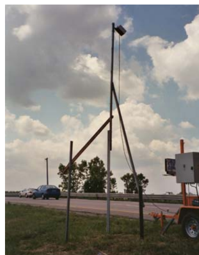
Photograph 7. Support Structure for Sensor When Installed in Depressed Medians (2003 Construction Season)
