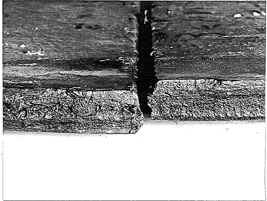
Figure 5. Weld which caused large brittle fracture in bridge. Note weld only at upper surface.
