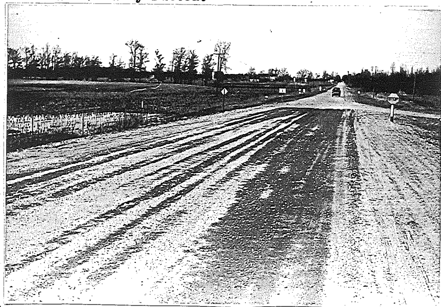
d. General surface condition at Station 248+00 Dark areas slightly rutted.
