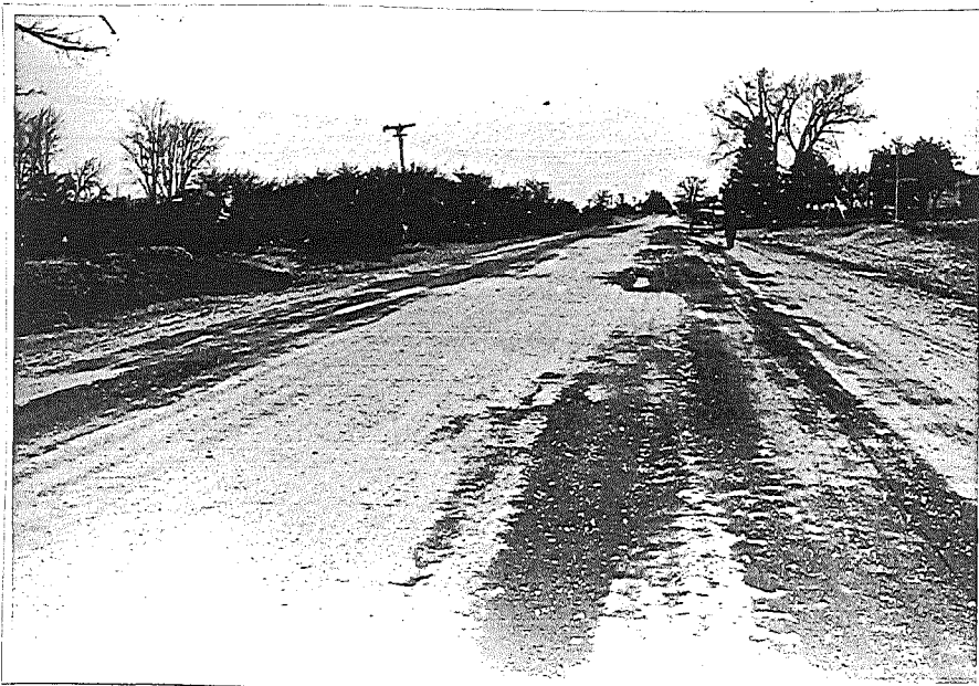
b. General surface condition Station 191+00 Dark areas badly rutted.
