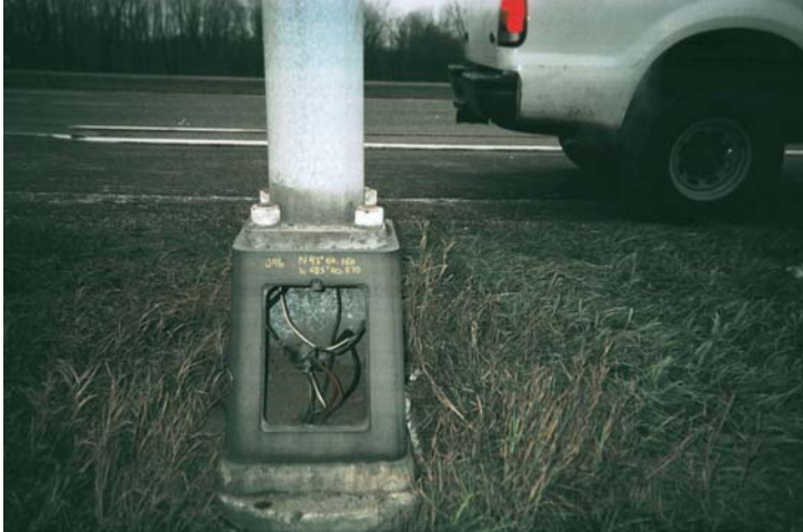
Figure 5. Missing access door.
