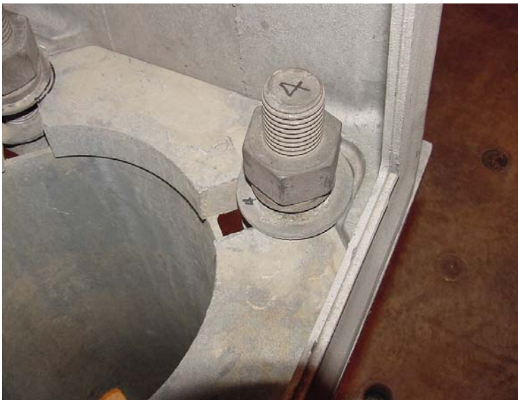
Figure 19. Reassembled Union Metal A2852 breakaway transformer base and Aluma-Form steel screw-in foundation assembly.
