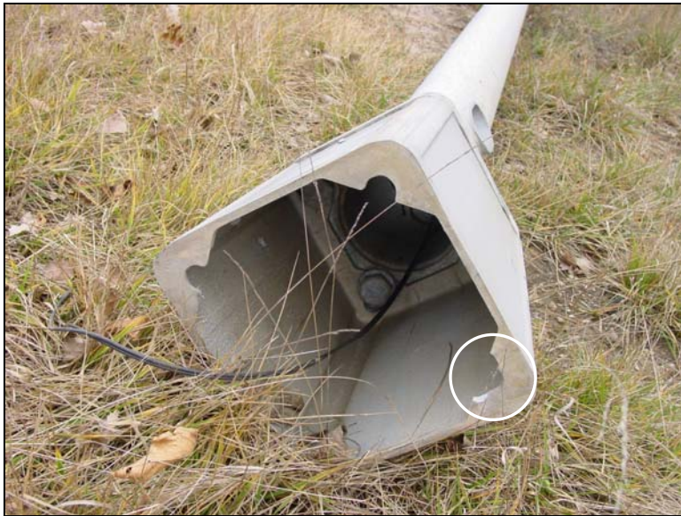
Figure 1. Toppled breakaway light standard that struck traffic
