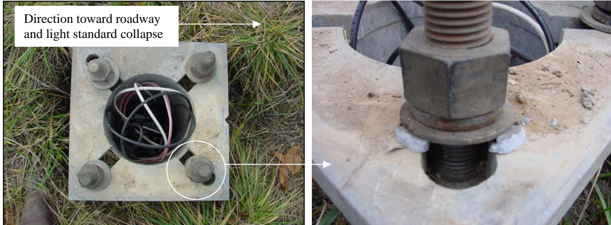
Figure 3. Steel screw-in foundation is shown on left and a close up of the broken breakaway transformer base tab on the right. Note the slot openings in the base plate of the steel screw-in foundation.
