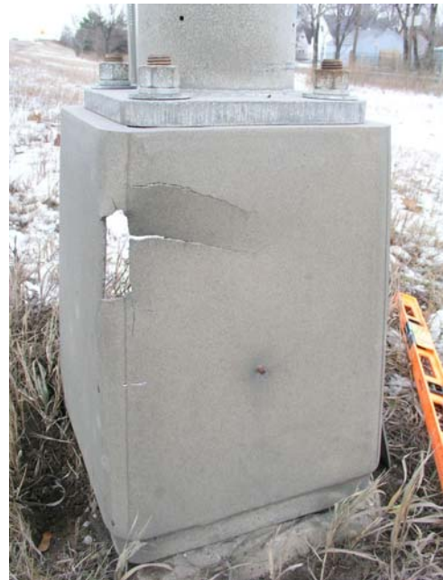
Figure 11. Damaged breakaway transformer base.
