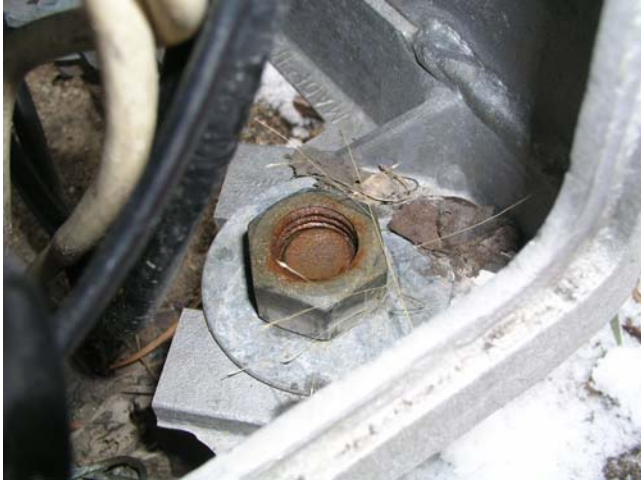
Figure 8. Incomplete nut engagement to the anchor bolt.
