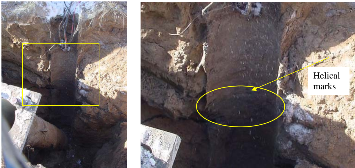
Figure 16. Steel screw-in foundation removal. The picture on the right is a close-up of the inset rectangle in the left photo.
