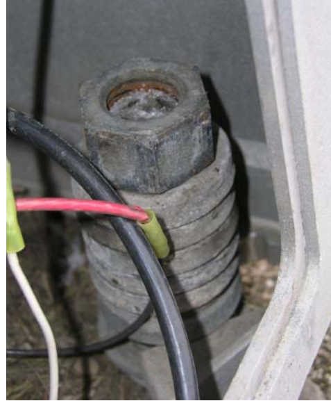
Figure 9. Stacked washers and incomplete nut engagement to the anchor bolt.
