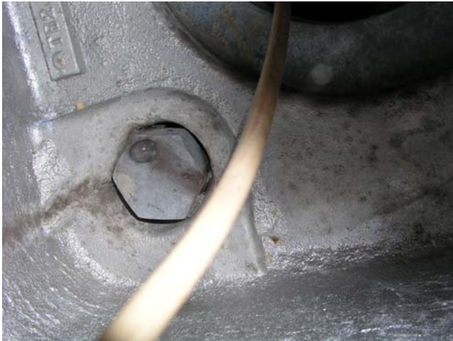
Figure 10. Replacement of top bolt assembly required due to missing washers.
