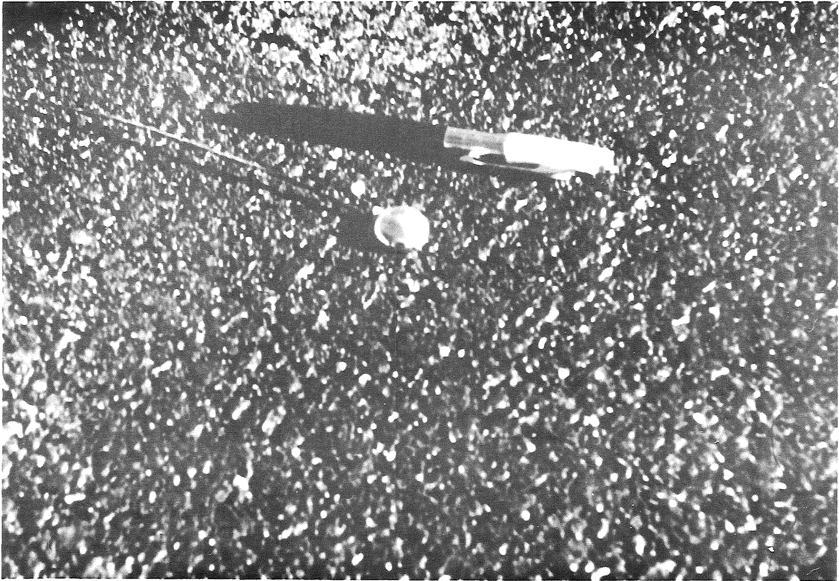
Figure 3. Showing a typical installation of the thermocouple wires using chair leg glides for supporting the ends of the wires.
