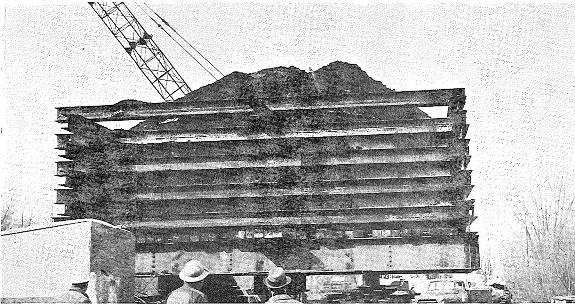
Figure 104. Movable reaction box at Muskegon, showing rollers, rail, and cribbing (upper left); test row (upper right foreground) with jack, dials, and reference beams in place; and reaction box filled with sand (lower left).
