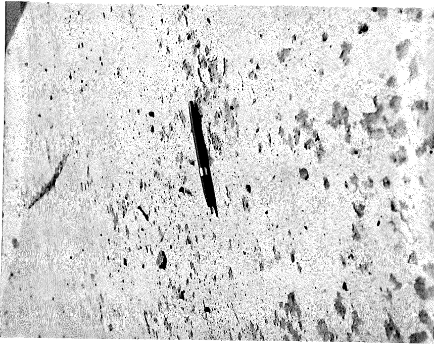
Figure 3. Typical pitting or light scale found on portions of refuge sidewalk pours.
