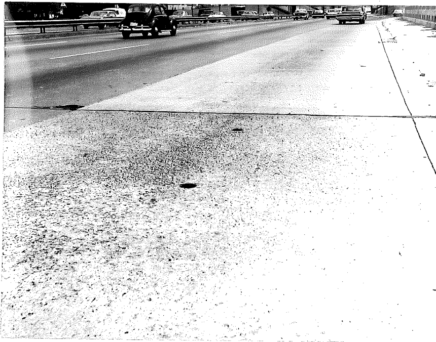
Figure 2. Heavy scaling at east end of Span 28 (cores 8 and 9). Lightly scaled surface of Span 29 in background.
