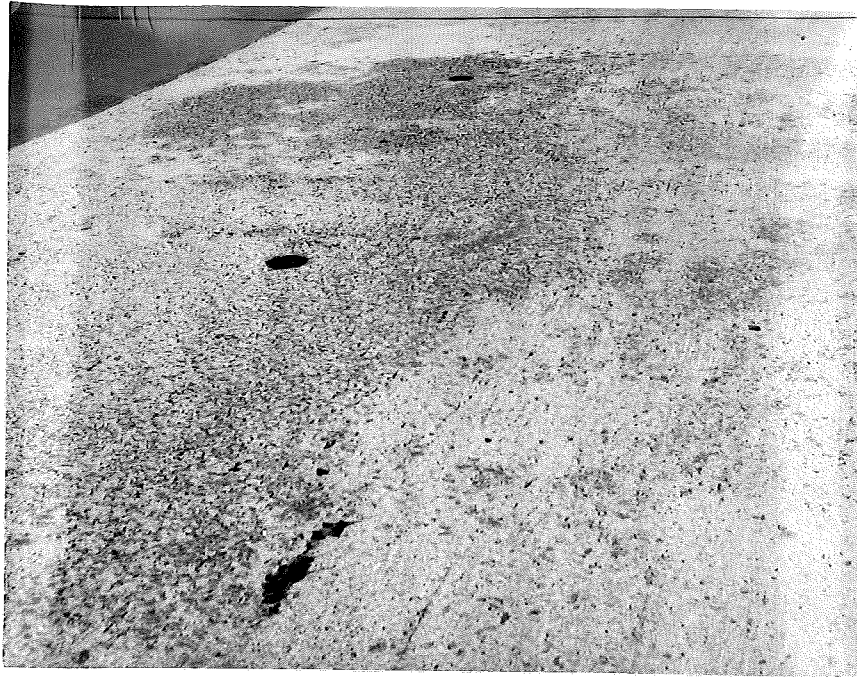
Figure 1. Variable scaling pattern at east end of Span 24 (cores 10 and 11).
