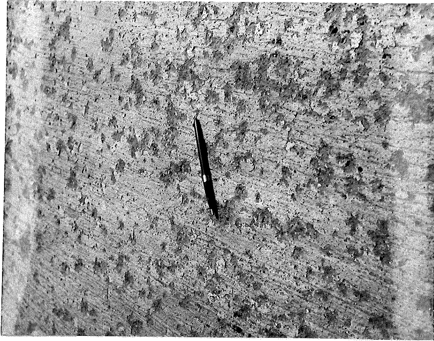
Figure 4. Typical light scale found in some roadway surface areas.
