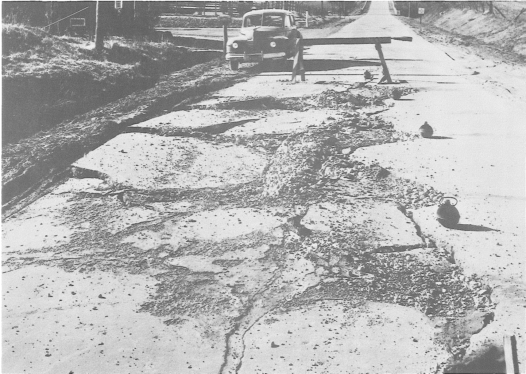
Figure 5. An extreme example of pavement damage resulting from frost action (furnished by Illinois Division of Highways).
