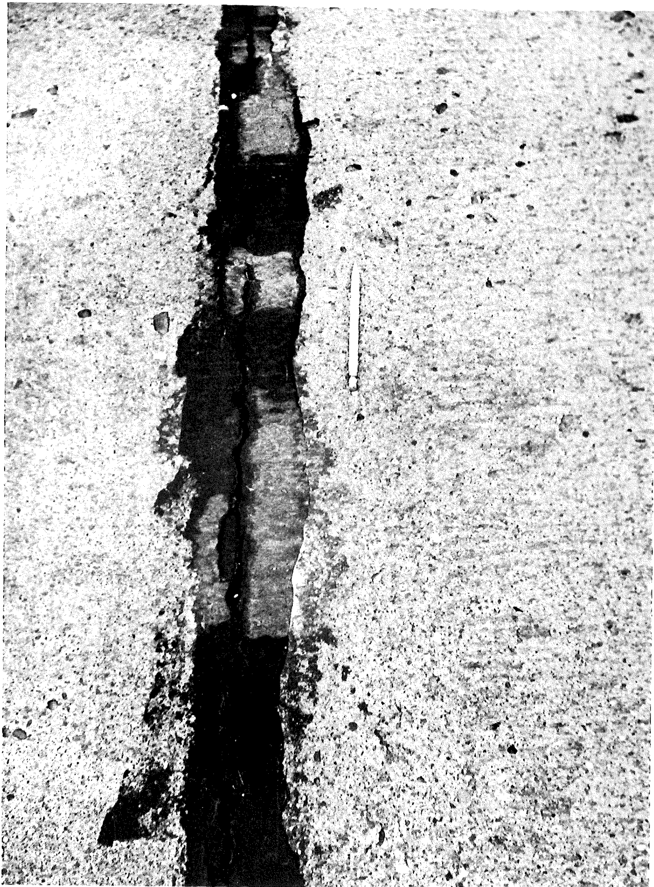
▲ STATION 187+00. EXPANSION JOINT SEALED WITH BRAND B. SEALER (SOA ASPHALT). COMPLETE ADHESION FAILURE BUT NOT MUCH COHESION FAILURE.
