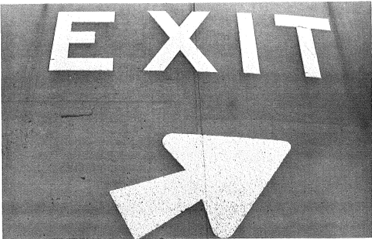
Figure 7. Typical condition of "Old" (above) and "Very Old" (below) signs on I 94.
