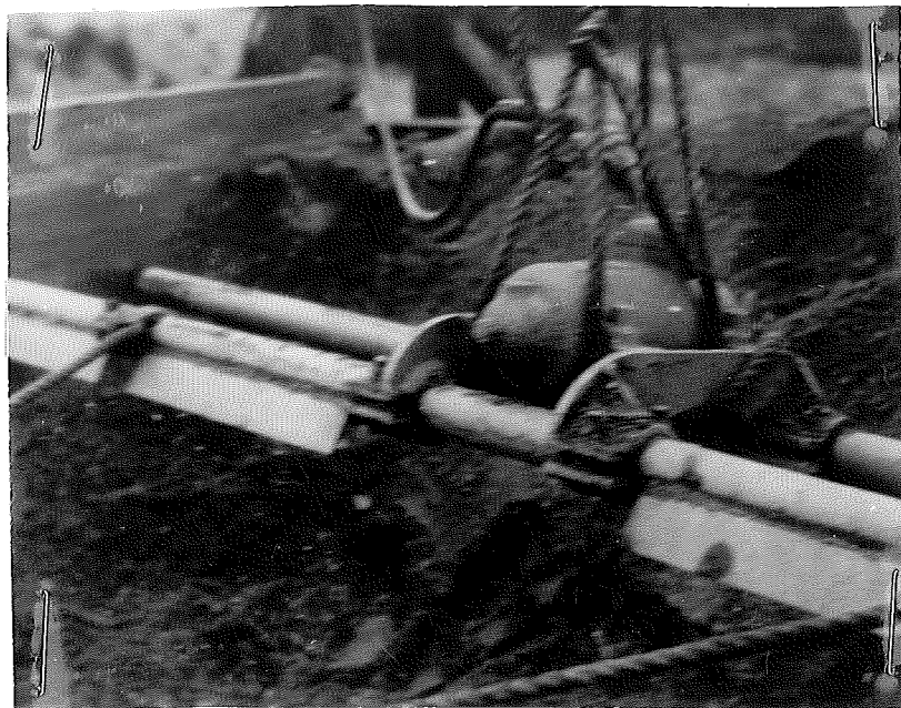
Figure 4. Vibratory Tubes actuated by Jackson PT-21A Vibrator Motor.
