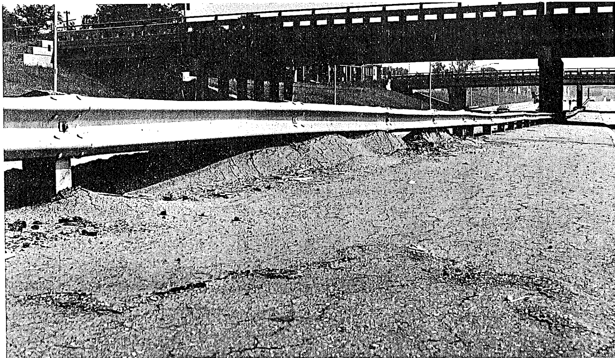
Figure 1. Distressed section of open hearth slag based median along the Fisher Freeway, I 75, Detroit.
