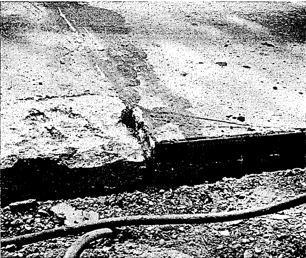
▲ Figure 2. A typical corner break with shoulder excavated to show details. First in a series showing steps in repair method.
