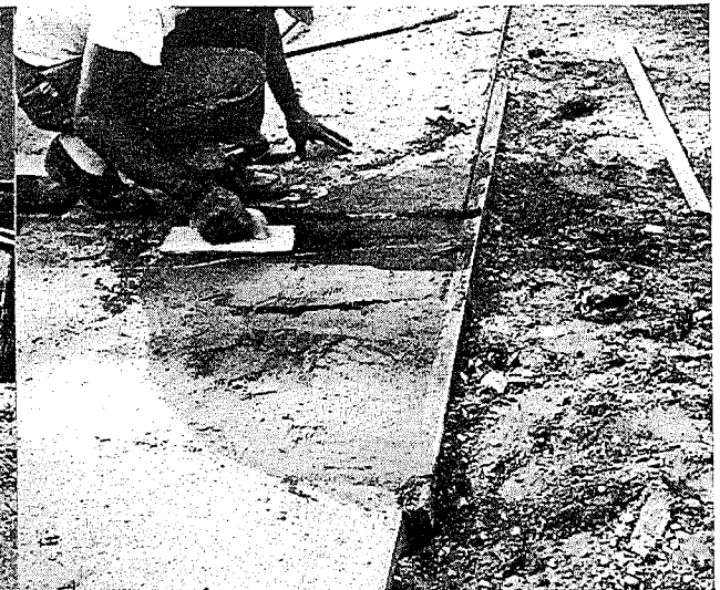
▲ Figure 12. Curing of a repaired corner break by covering with Sisalkraft paper.
