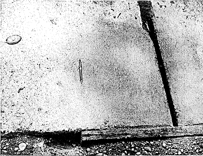
Figure 13. A typical repaired corner break.
