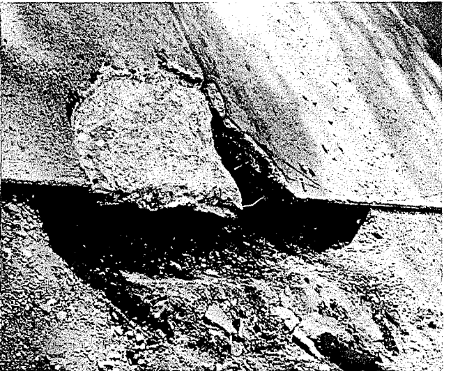
▲ Figure 3. Close-up of lower break in Figure 2 with loose and decomposed material removed.
