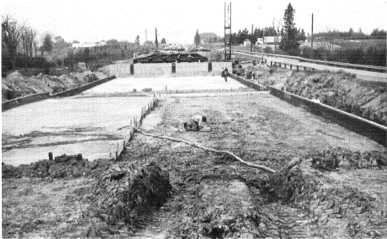
Figure 4. Fill divided into sections small enough to be poured in 8 hours or less.
