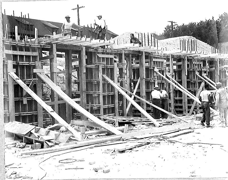
Form work under present practice using standard timber wales for concrete column construction.
