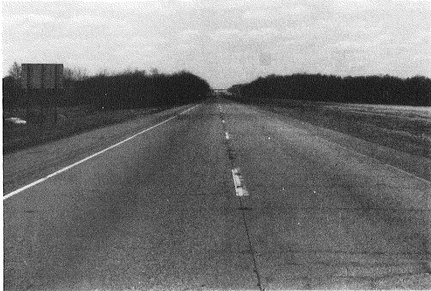
Figure 11. The longitudinal joint in the CRCP test sections exhibited only minor to moderate spalling and patching and only occasional areas where the joint had separated.
