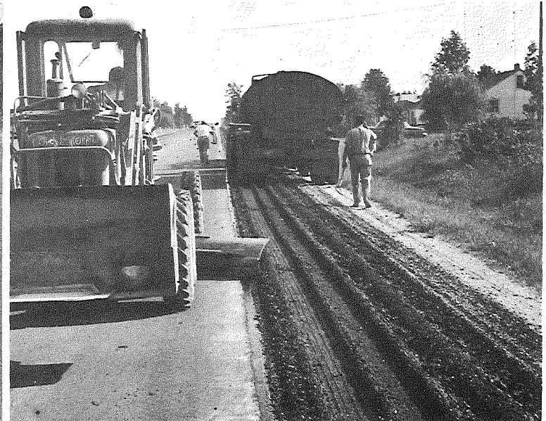
Figure 14. Loose shoulder material during curing of asphalt-aggregate mixture.
