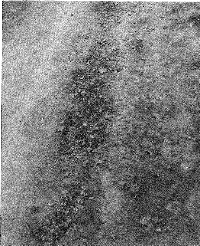
Figure 6. Loose condition of soil cement surface before sealing. Note presence of stones.
