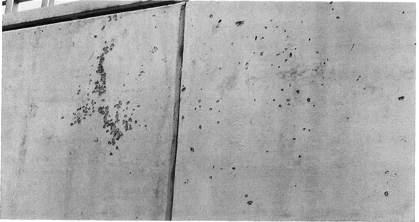
Figure 12. Scaling or pitting similar to that on the railing posts has occurred on the south retaining wall between the separate roadways, probably due to splashing of chemical-laden slush and snow by passing vehicles and winter maintenance operations. Sept. 1960.
