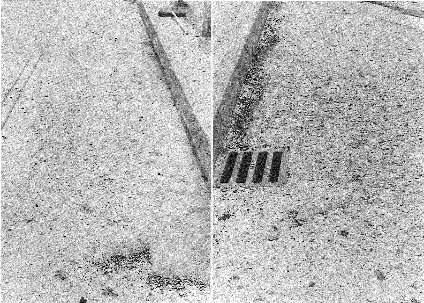
Figure 2. Scaled deck pavement on northbound roadway -- passing lane at center of Span 1 (left) and traffic lane at south end of Span 3 (right). Sept. 1960.
