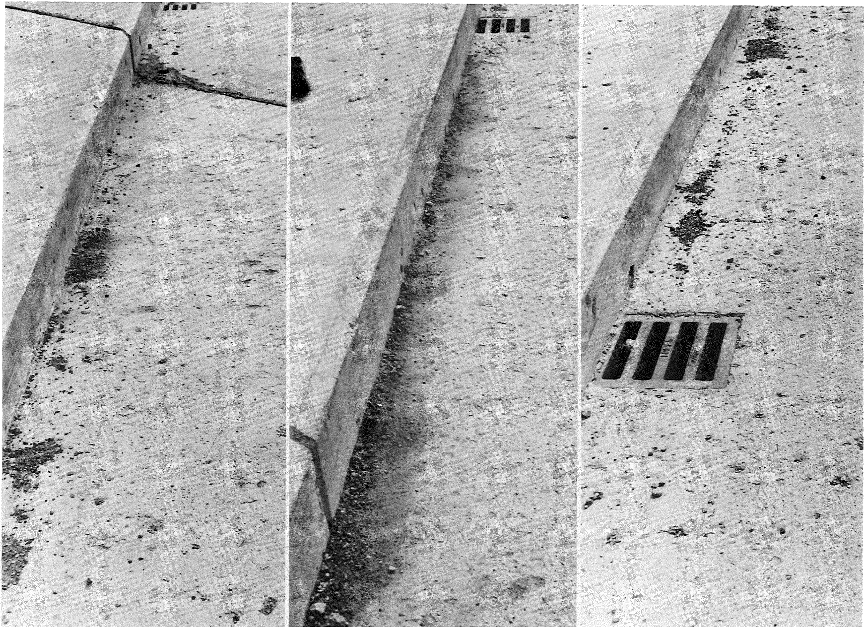
Figure 3. Scaled deck pavement on Span 4, northbound roadway traffic lane -- south end (left), center (center) and north end (right). Sept. 1960.
