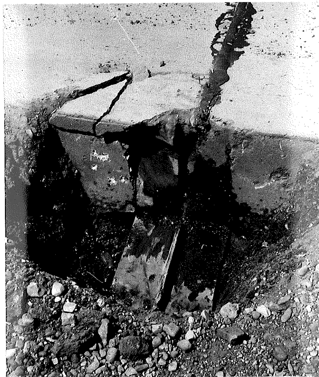
Figure 3. End plate distorted, with one corner embedded in concrete, resulting in edge break; before (above) and after (below) bending down end plate. Sta 874+10
