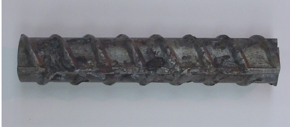
Figure 5 MMFX reinforcement directly exposed to salt solution
