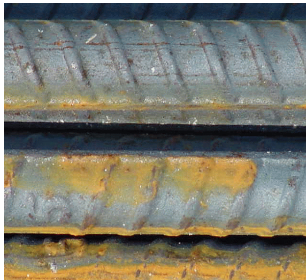
Figure 6 Mill scale on MMFX reinforcement, R01 of 82022
