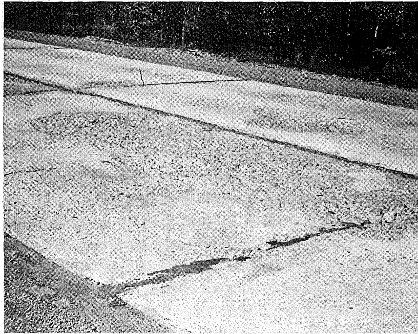
Fig. 8. Typical scaling and pitting at Sta. 34/00.
