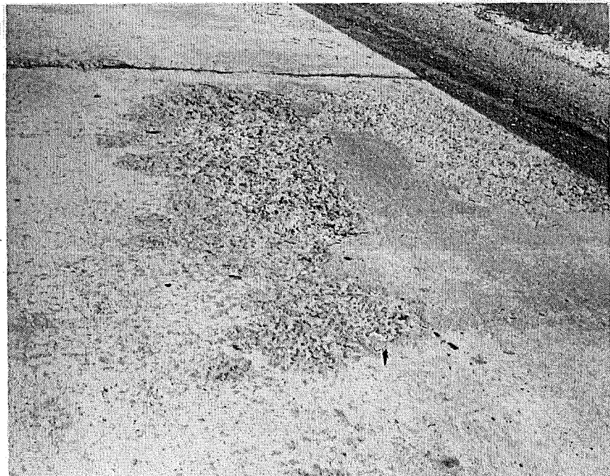
Fig. 7. Character of scaling and deep pitting 33+00
