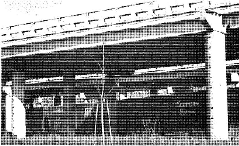
Figure 1. Location of instrumentation and view of instrumented span.
