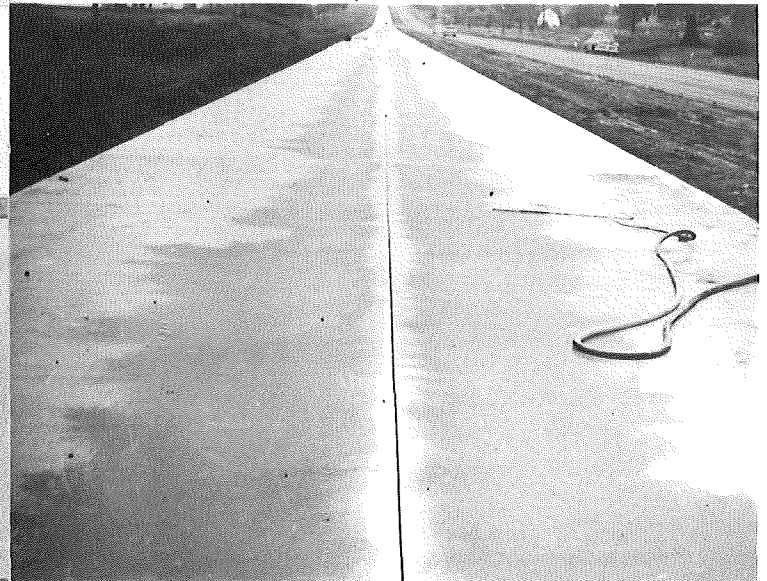
FIGURE 5. SHOWS LONGITUDINAL CENTER JOINT AFTER CUT HAS BEEN MADE, BUT PRIOR TO SEALING.
