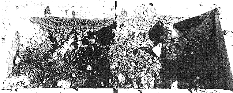
Figure 6. Deteriorated concrete in bottom of repair area.
