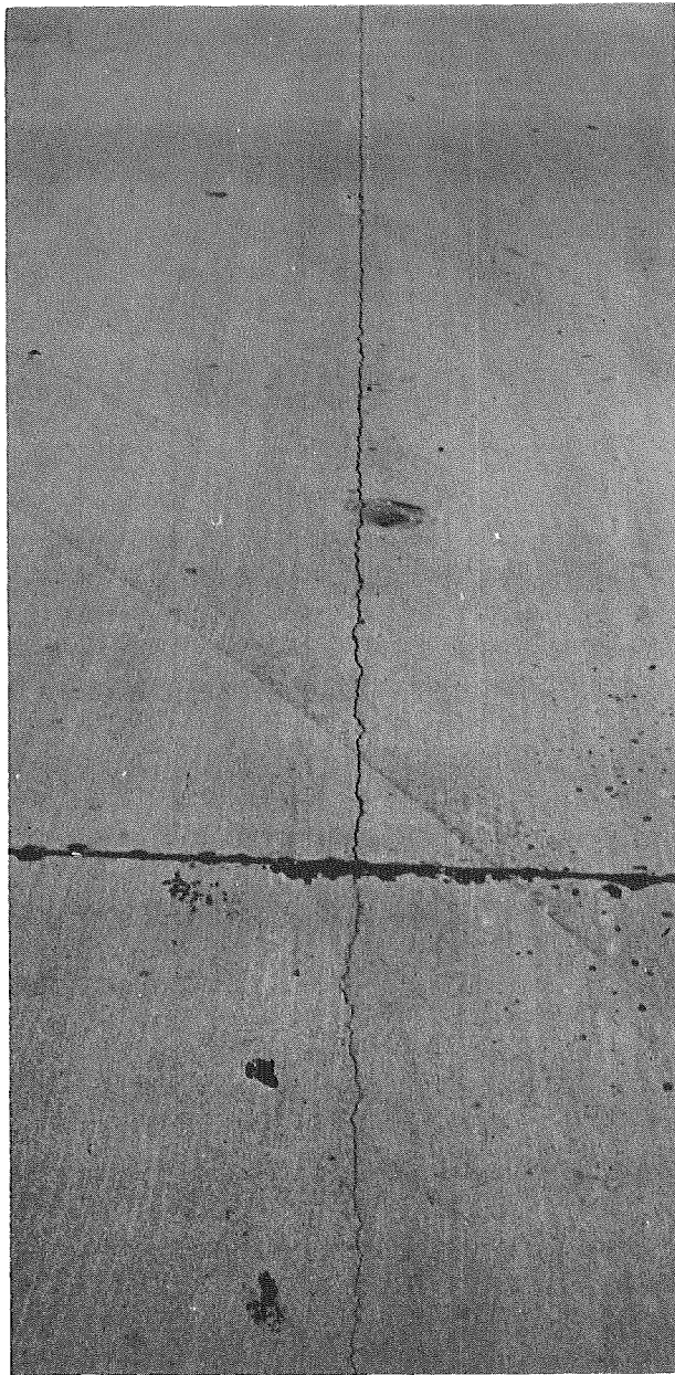
Figure 3. Condition of joint in standard pavement on Ill. 131. Note zig-zag appearance.
