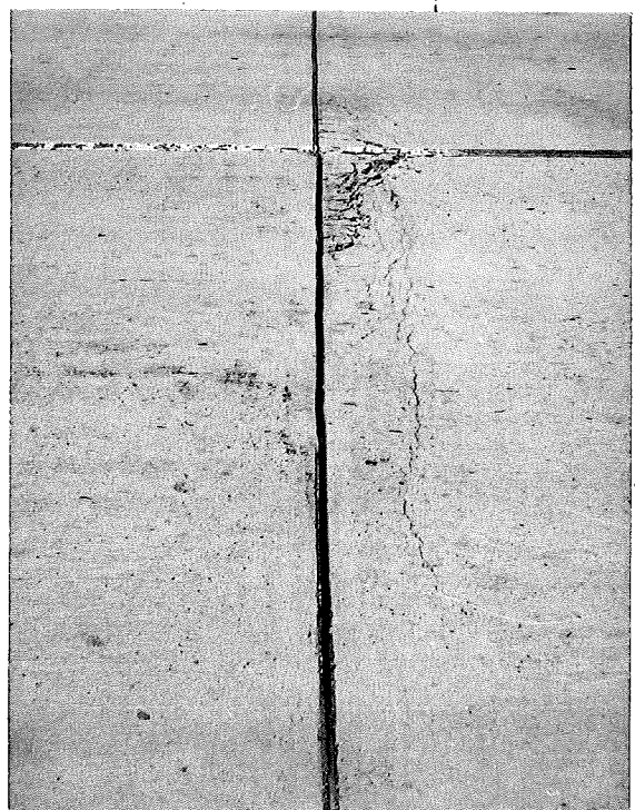
▲ FIGURE 8. THE SAME JOINT, JUNE 9, 1954. SHOWING ADDITIONAL SPALLING WHICH HAS TAKEN PLACE SINCE THE 1953 SURVEY.
