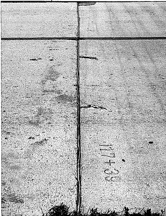
▲ FIGURE 3. SHOWING PAVEMENT CONDITION AS OF AUGUST 3, 1953. STATION 117+39. LOOKING EAST TO WEST.
