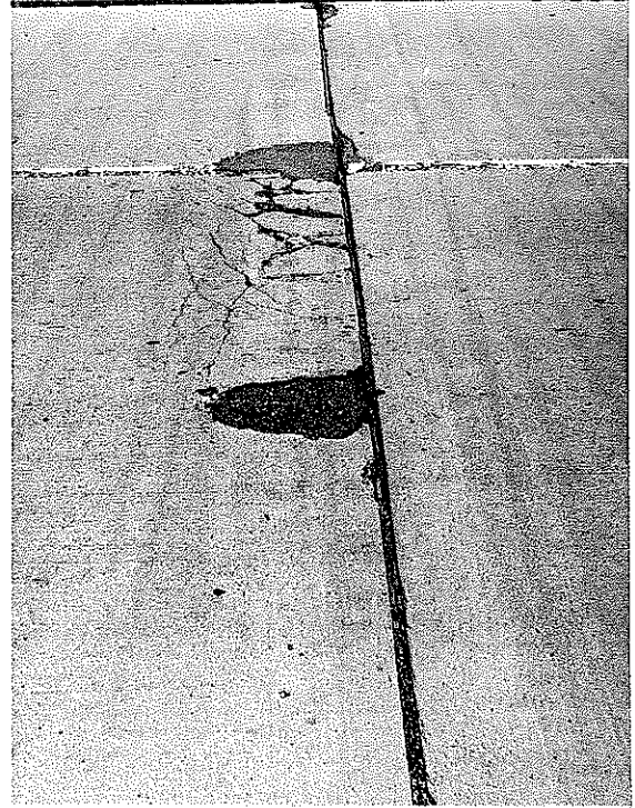
▲ FIGURE 2. THE SAME JOINT, JUNE 9, 1954. SHOWING PROGRESSIVE CHECKING WHICH HAS OCCURRED SINCE 1953 SURVEY.
