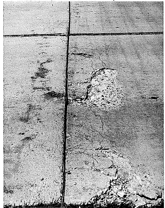
▲ FIGURE 4. THE SAME JOINT, JUNE 9, 1954. NOTE THE GREAT INCREASE IN DISINTEGRATION OF THE SLAB WHICH HAS TAKEN PLACE SINCE 1953 SURVEY.
