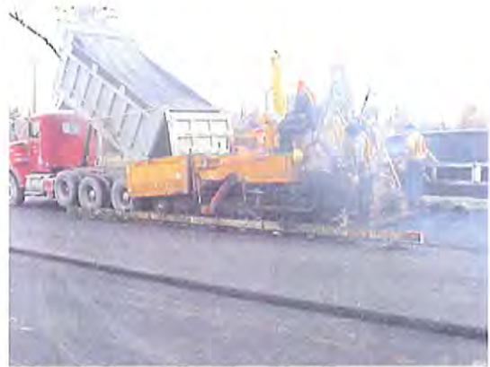
Figure 7. Grade control used for middle two lanes. Note wheeled ski on right side behind the paver.
