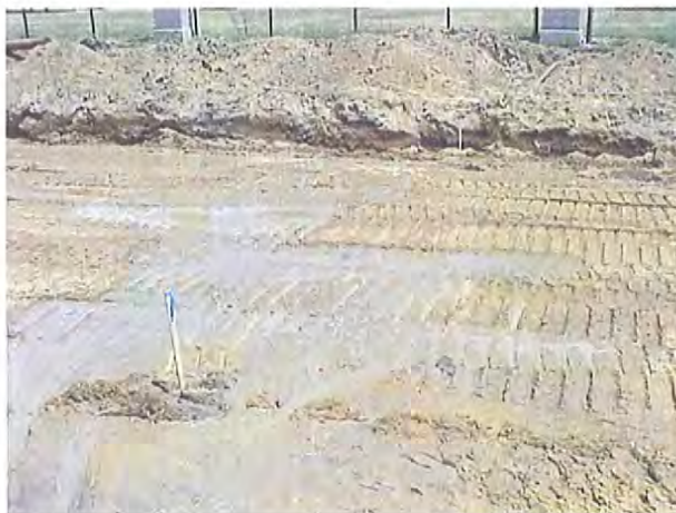
Figure 8. Saturated soil condition in test section 2 created by leaking water main valve.
