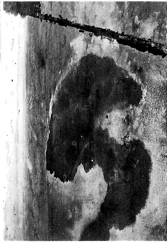
Figure 2. Spalled area over high steel after chipping (top), and after about four hours of traffic (bottom). The patched lane was closed for one hour after placement. Northwest corner of passing lane, US 127 bridge over NYC RR, north of Jackson (5-17-66).
