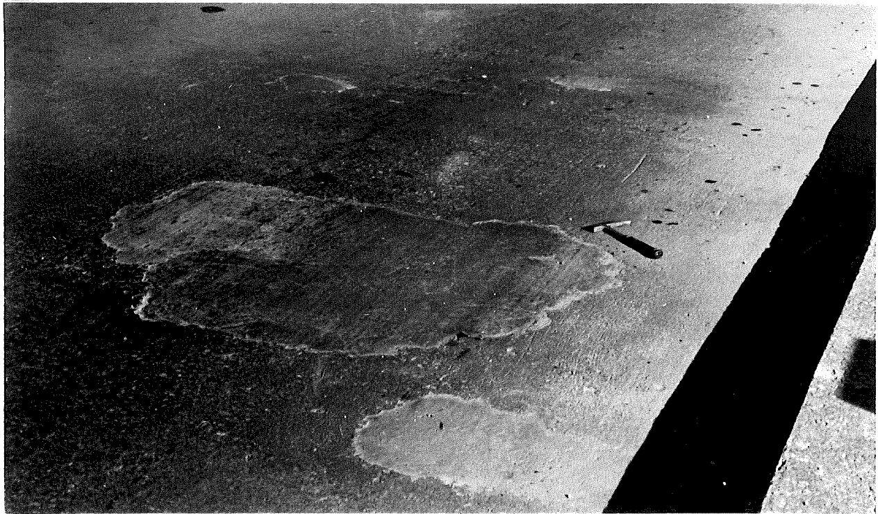
Figure 4. Two patches near east curb, toward north end of S. Pennsylvania structure over NYC RR, Lansing (9-8-66).
