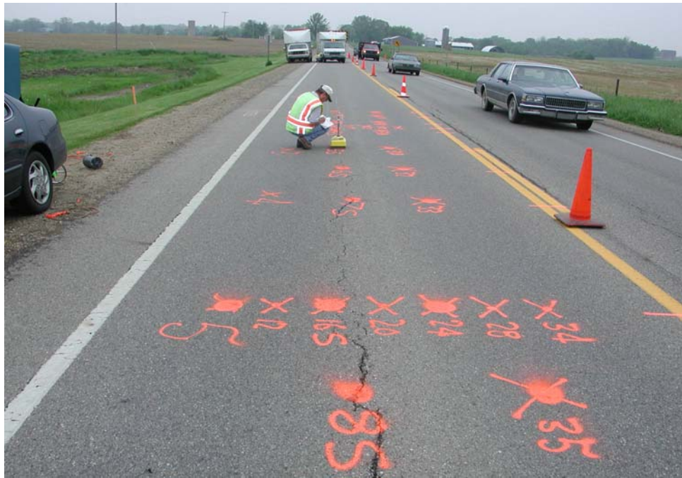
Figure 4.9 TDC in segregated areas on M-50 test section 2 (flexible pavement)
