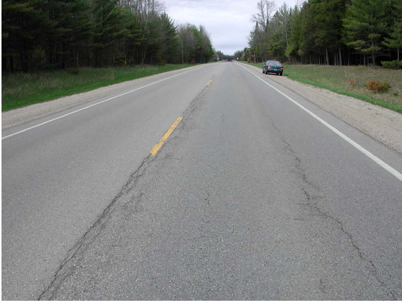
Figure 2.1 Top-down cracks in a rubblized pavement (US-131)
