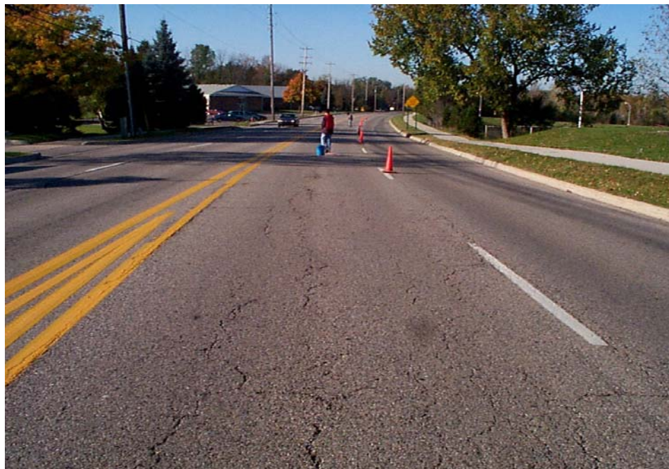
Figure 4.13 TDC in heavily segregated areas on Marsh Road (flexible pavement)
