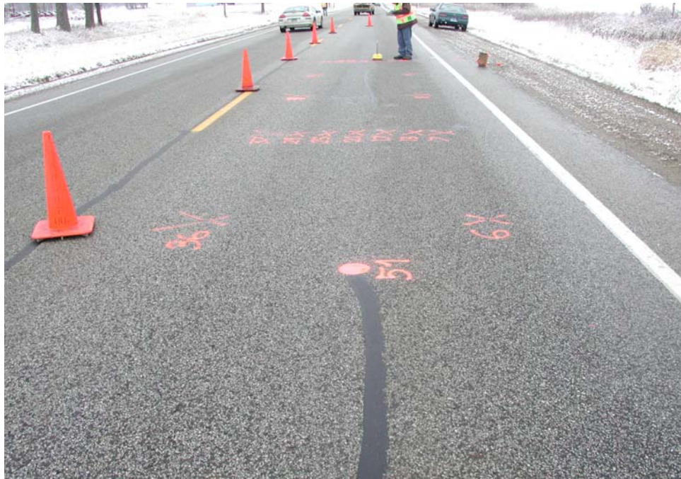
Figure 4.11 TDC in segregated area on M-50 test section 2 (flexible pavement)
