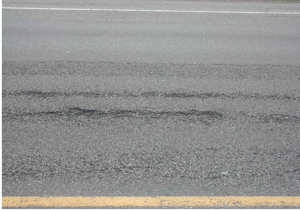
Figure 4.4 TDC and raveling in heavily segregated areas on US-23, May 2002, 2 years after construction (rubblized pavement)
