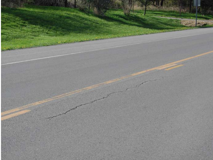
Figure 4.16 Longitudinal TDC at the edge of the wheel path on US-23, control section 01052 job number 32335 BMP
