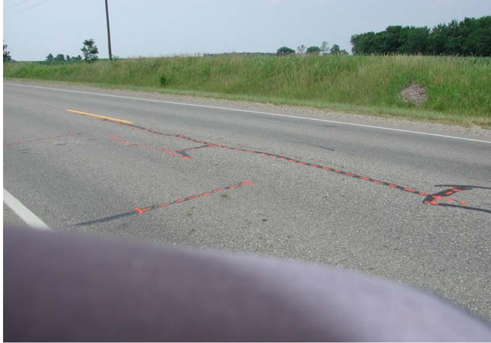
Figure 4.8 TDC in segregated areas on M-50 test section 1 (flexible pavement)
