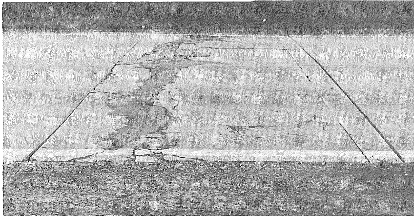
Figure 2. Transverse saw limits. The second saw cut, about 8 in. inside the repair limits at one end, was made to facilitate removal of the distressed pavement.
