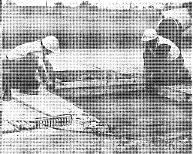
Figure 13. The elevation of the cement mortar was established by a template in a manner similar to that used for subbase elevation.
