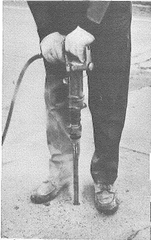
Figure 5. Drilling 1-1/4-in. diameter holes, full-depth, for insertion of lift pins. Three holes were drilled in each half-lane slab to be removed.
