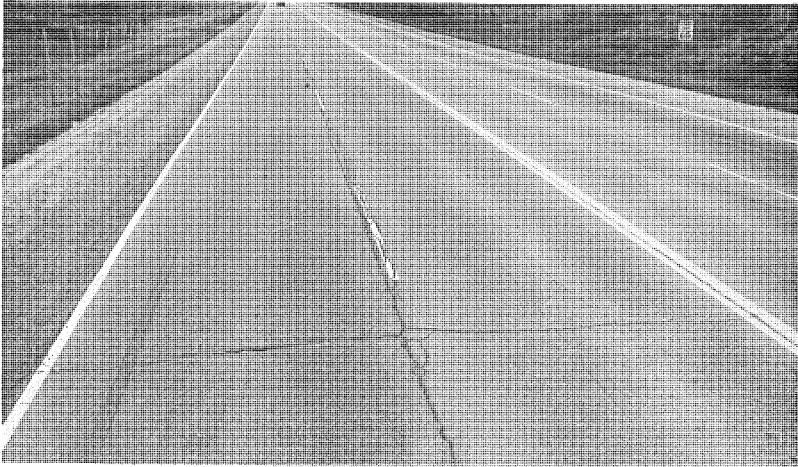
Figure 8. Markings ( (f) type) looking S on US 27, S of Clark Rd after two years of service. The NB lane lines (left) are affected by reflection cracking of the bituminous surface (9-14-71).
