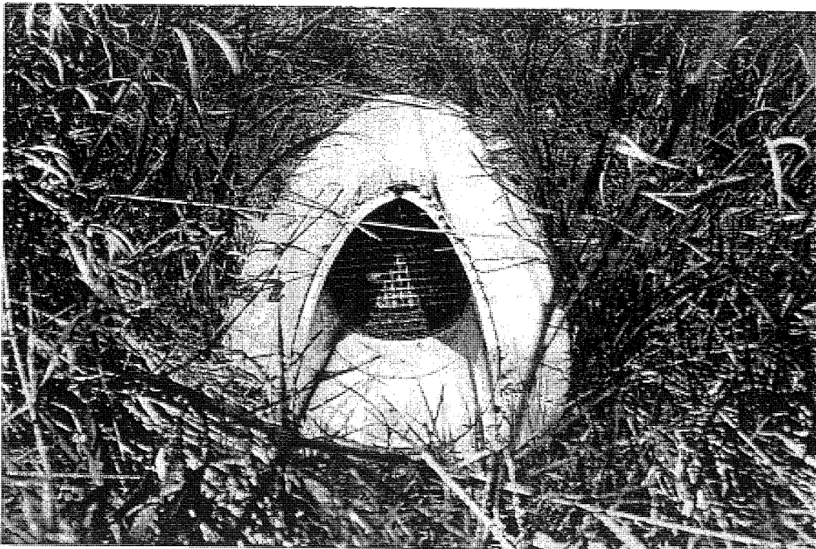
Photo C4. A typical drainage structure of CSN# 11017-32516A (Section A), EB. Water can be seen flowing freely from the drain after coring.
