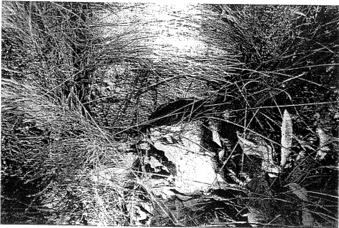
Photo C44. A drainage structure that is clogged with sand and debris on CSN# 77023-21586A EB.
