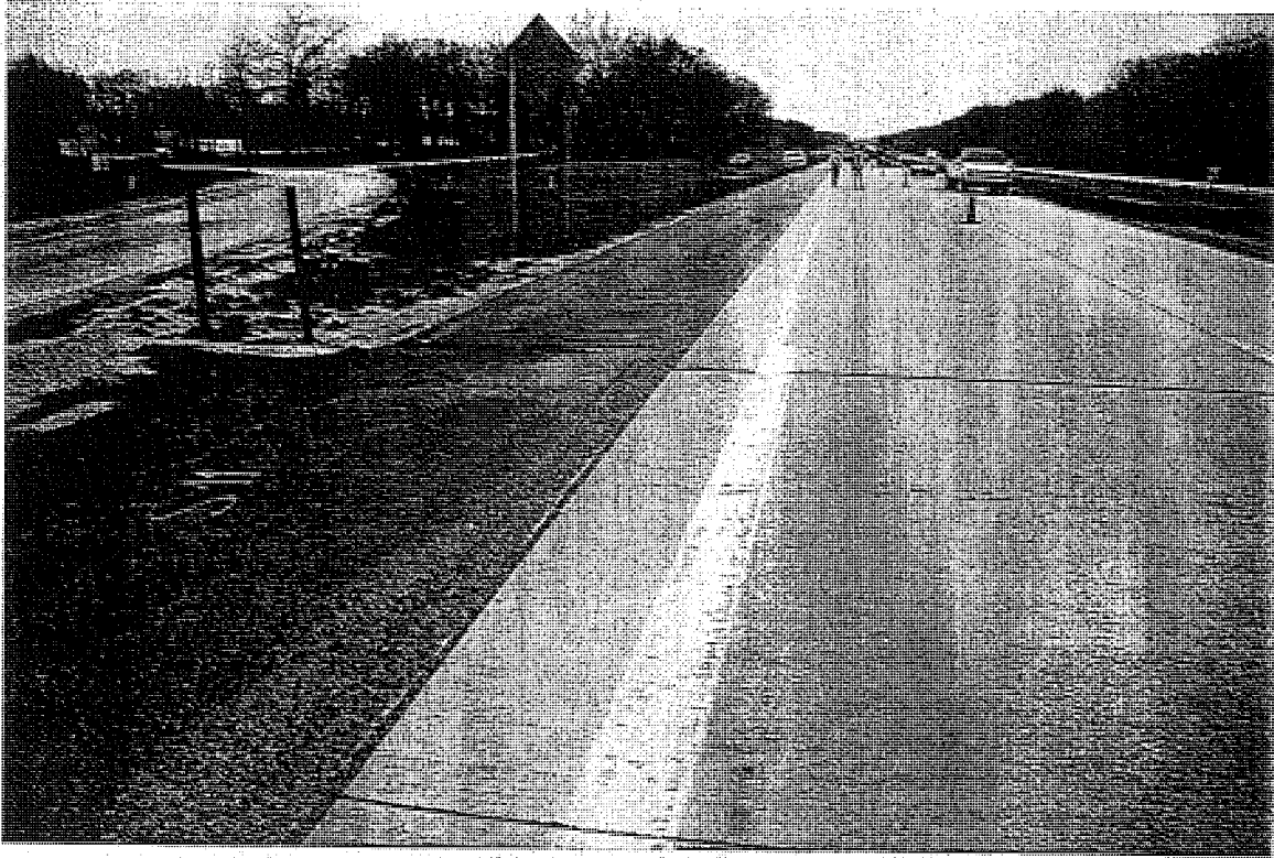
Photo C5. An overview looking west on CSN# 11017-32516A (Section C), EB. This section has a 14 ft widened truck lane and an asphalt shoulder. Transverse joint spacing varies from 15 to 17 ft.
