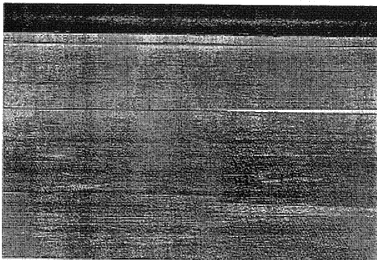
Photo C18. A typical tight mid-slab crack on CSN# 19042-02233A (Section C) EB the crack propagates from the shoulder into the truck lane.
