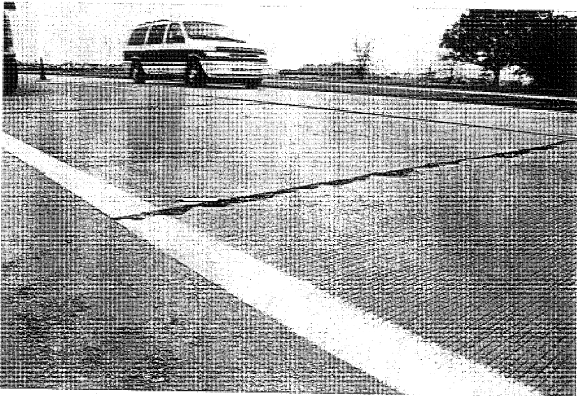
Photo C46. A severely spalled and faulted transverse crack in CSN# 77024-20821A (Section A), EB.
