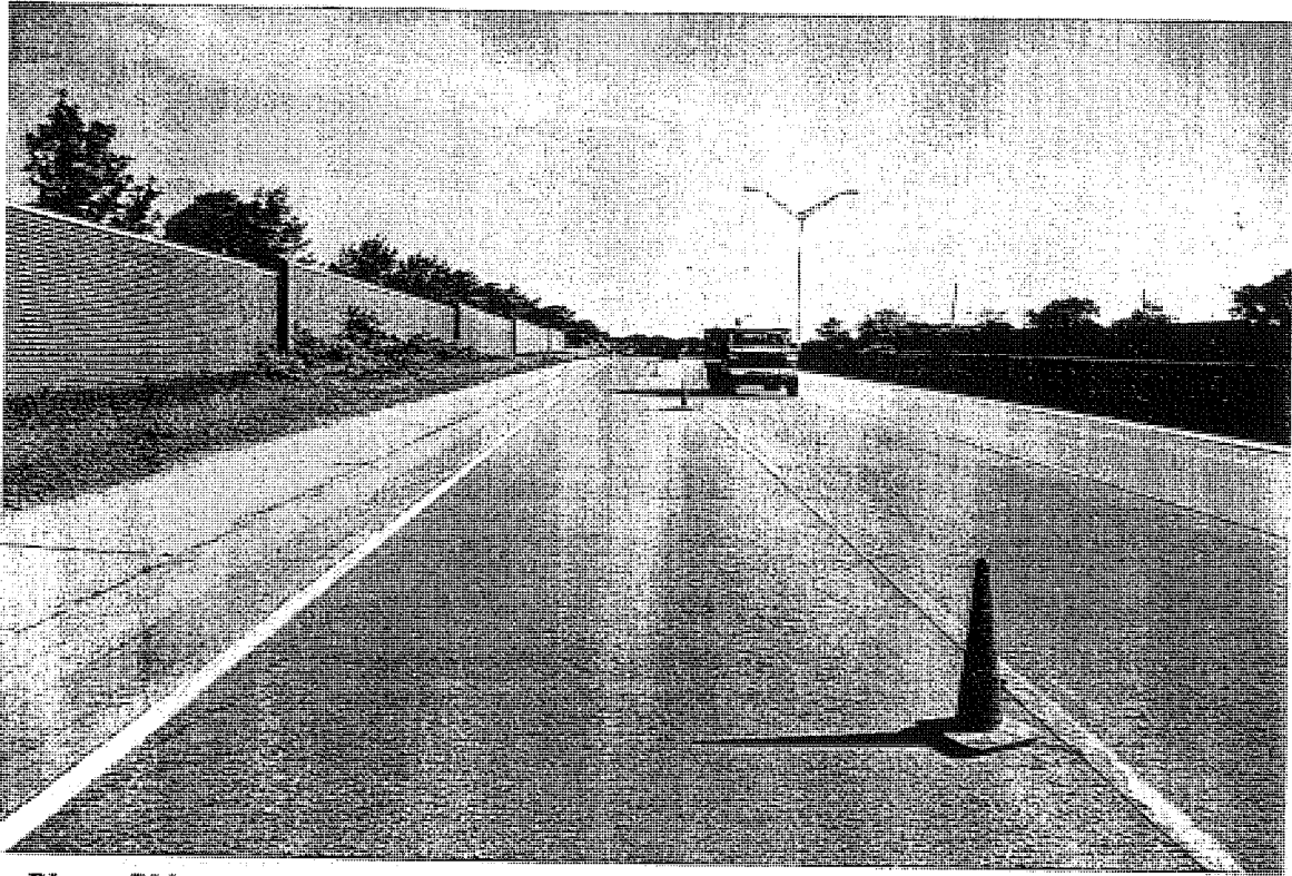
Photo C29. An overview looking north on CSN# 25132-06582A SB. This photo shows the 3 lanes of traffic and the third point intermediate shoulder joints. The slab length is 44 ft in the driving lanes.
