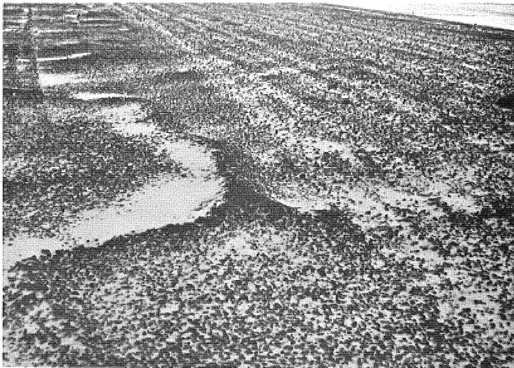
Figure 3. Unpaved parking lot at Detroit-Wayne Metropolitan airport.
