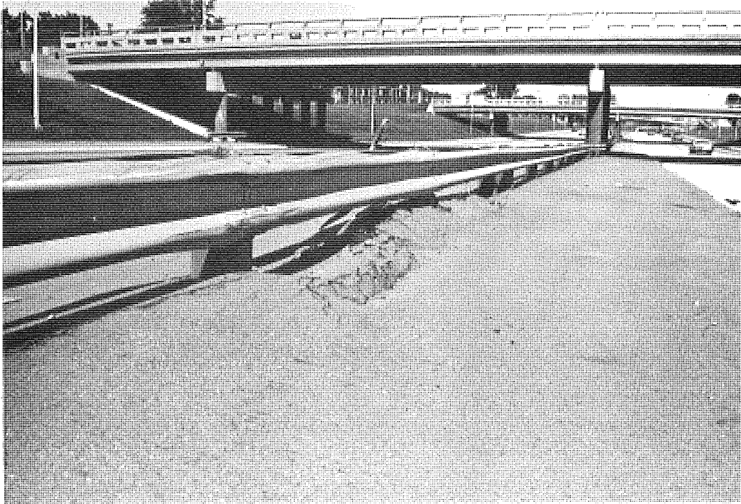
Heaving and buckling of bituminous surface
