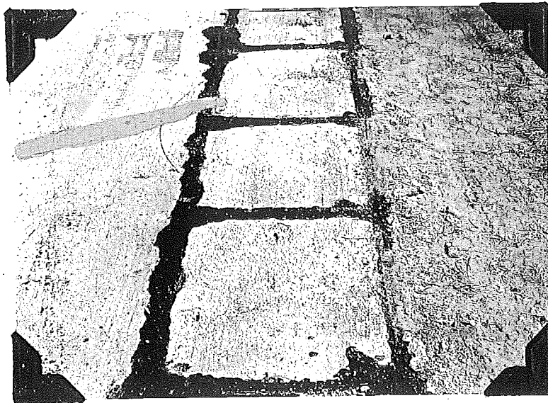
Figure 4B. Calcium chloride panel of test area No. 2 after 26 cycles. Pavement 4 years old containing cement brand No. 2. Project 18-20,C3. Station 500+50. 11 percent scaled.
