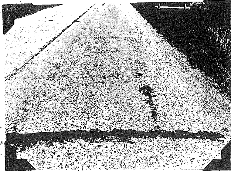
Figure 6. Photograph showing the effect of chloride salts on concrete containing inferior aggregates.
