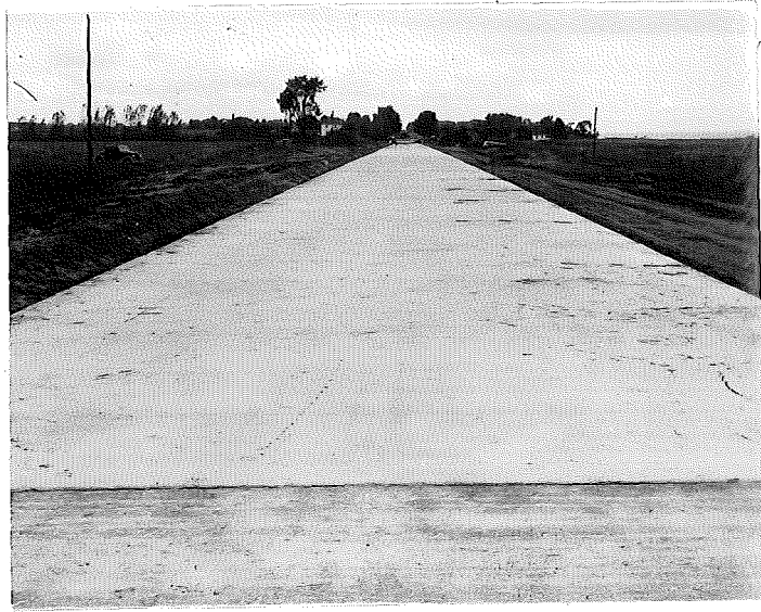
Figure 3. First day's pour immediately after removing forms on following morning, north Cree Station 1057+62.
