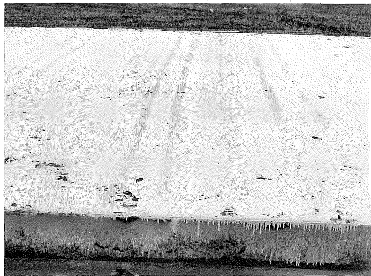
Figure 7. Ridging due to clogging of old type nozzles. This section was sprayed after dark. Station 1081+00.
