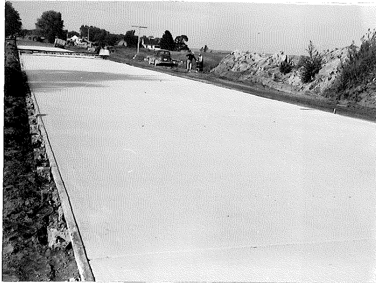
Figure 7. View of beginning of second day's pour. Application by double pass, using new nozzles with screens removed and spray bar slightly raised. Station 1066+71.
