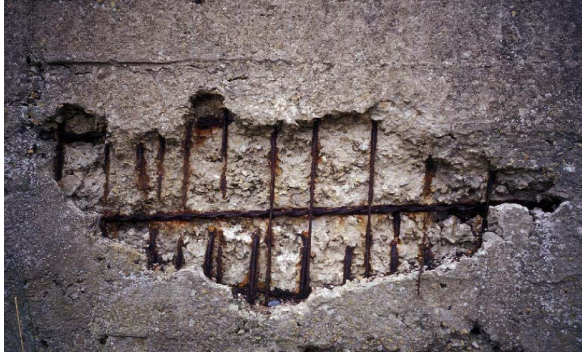
Figure 1.1 Steel Corrosion in Concrete
