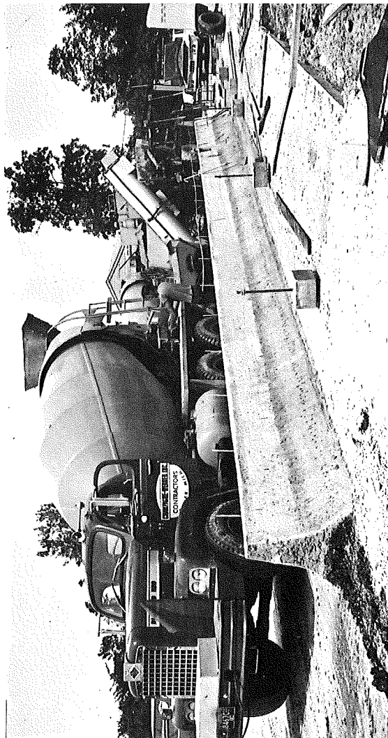
Figure 2. Median barrier ready for placement of concrete glare screen. Note that longitudinal reinforcement has been left out of the section in the foreground.
