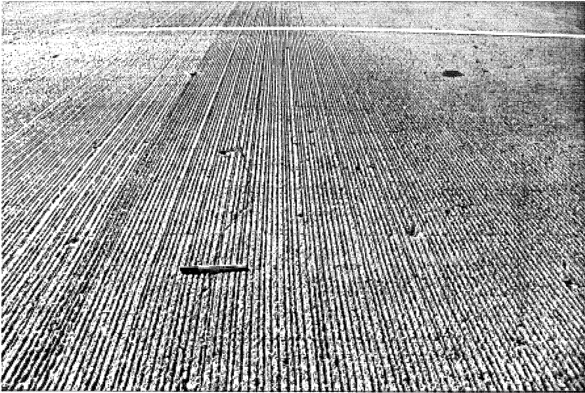
Photo C27. A midslab crack along CSN# 19043-02234A, WB. The crack propagates from the intermediate shoulder joint, which is typical for this section.
