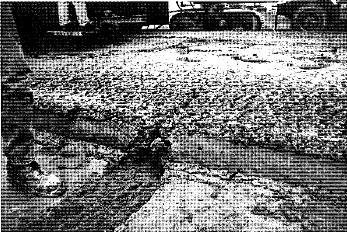
Photo C39. A view of the thermocouple rig immediately after installation in CSN# 47065-28215A WB. The rig is installed between paving lifts, and the cables are buried to protect them from damage during the second paver pass.
