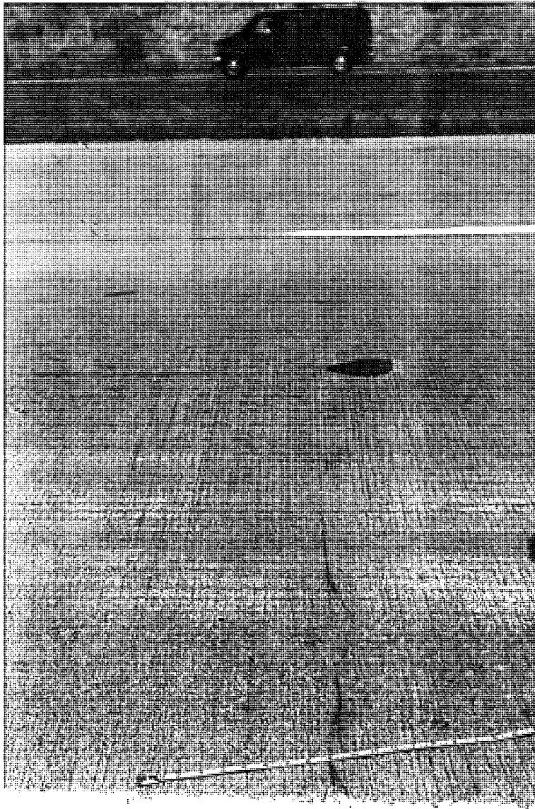
Photo C19. A tight crack on CSN# 19042-02233A (Section C) EB, joints are in good condition as can be noted here.
