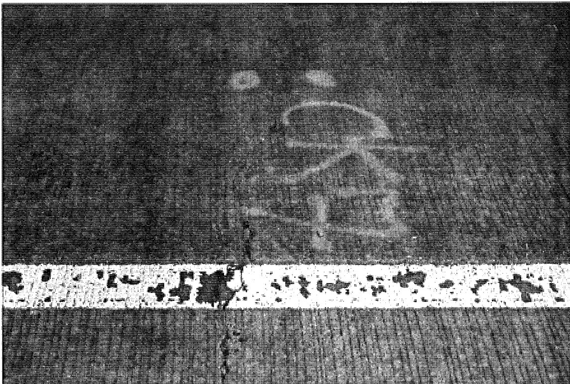
Photo C2. A typical midslab crack on CSN# 11017-32516A (Section A), EB. The beginning of some spalling can be seen at the bottom of the photo.
