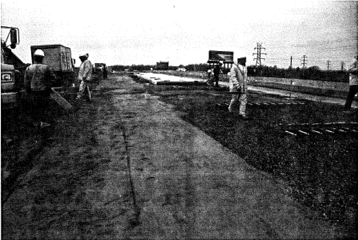
Photo C37. An overview of CSN# 47065-28215A WB looking west, just prior to paving. The open graded drainage course and dowel cages are visible.
