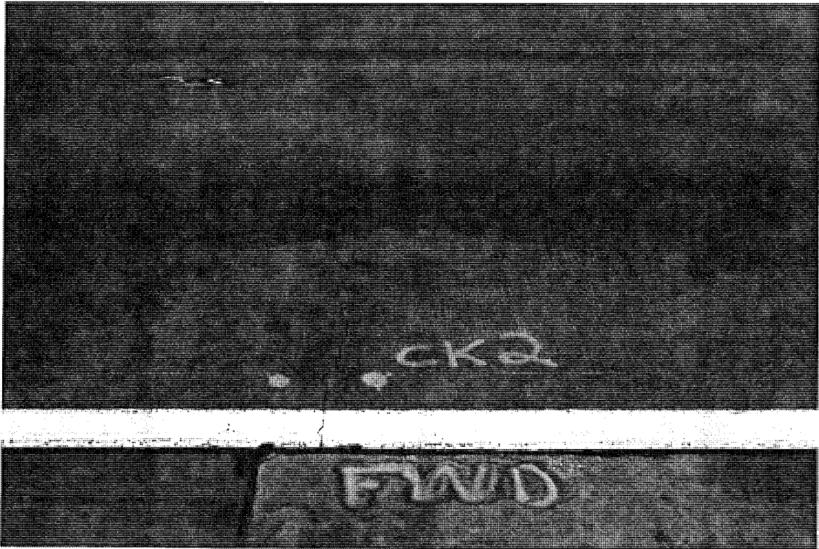
Photo C51. A tight transverse crack induced by the intermediate shoulder joint on CSN# 77024-17988A, (Section B), EB.
