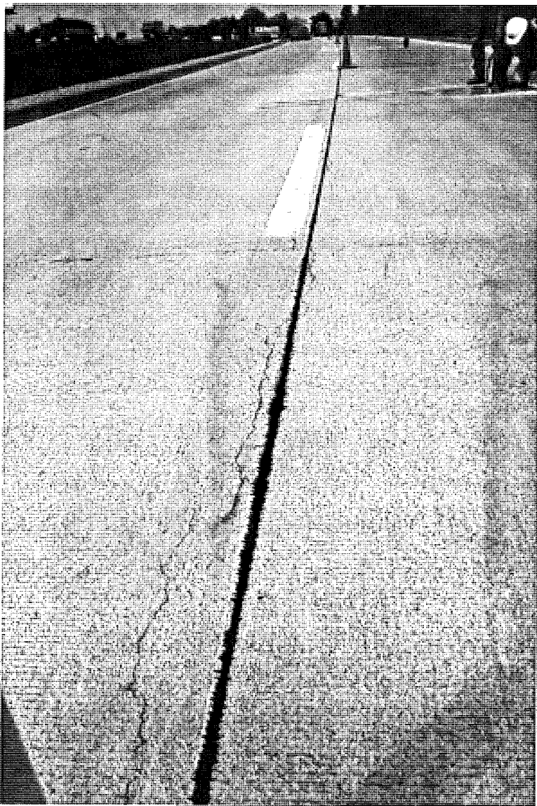
Photo C9. An overview looking west on CSN# 11017-32516A (Section D), WB. A tight longitudinal crack running parallel to the longitudinal joint can be seen.
