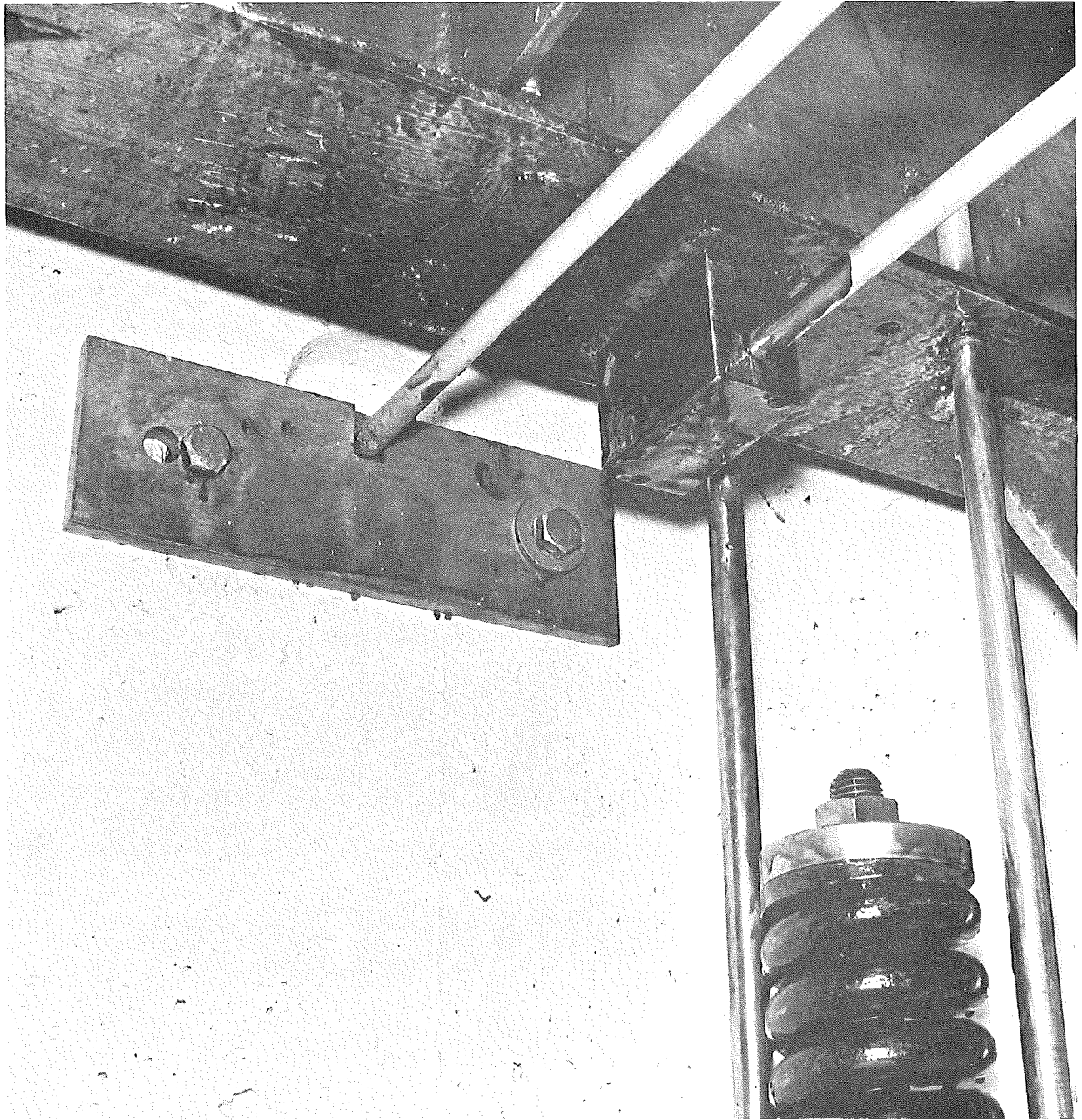
Figure 5. Platform transverse anchor rods showing one wall anchor and one rod-to-platform attachment block.
