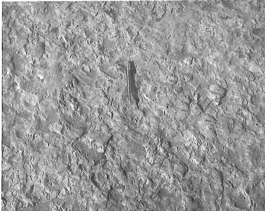
Figure 7. Close view of scaled surface. Note smooth texture of coarse aggregate particles.
