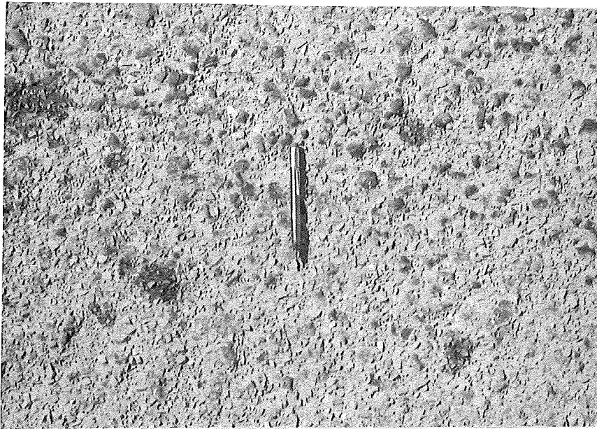
Figure 17. Texture of surface at last area 19. Project CS 53-26, C2.
