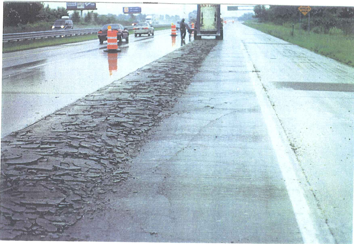
Showing pavement being broken by Guillotine Breaker prior to removal by backhoe
