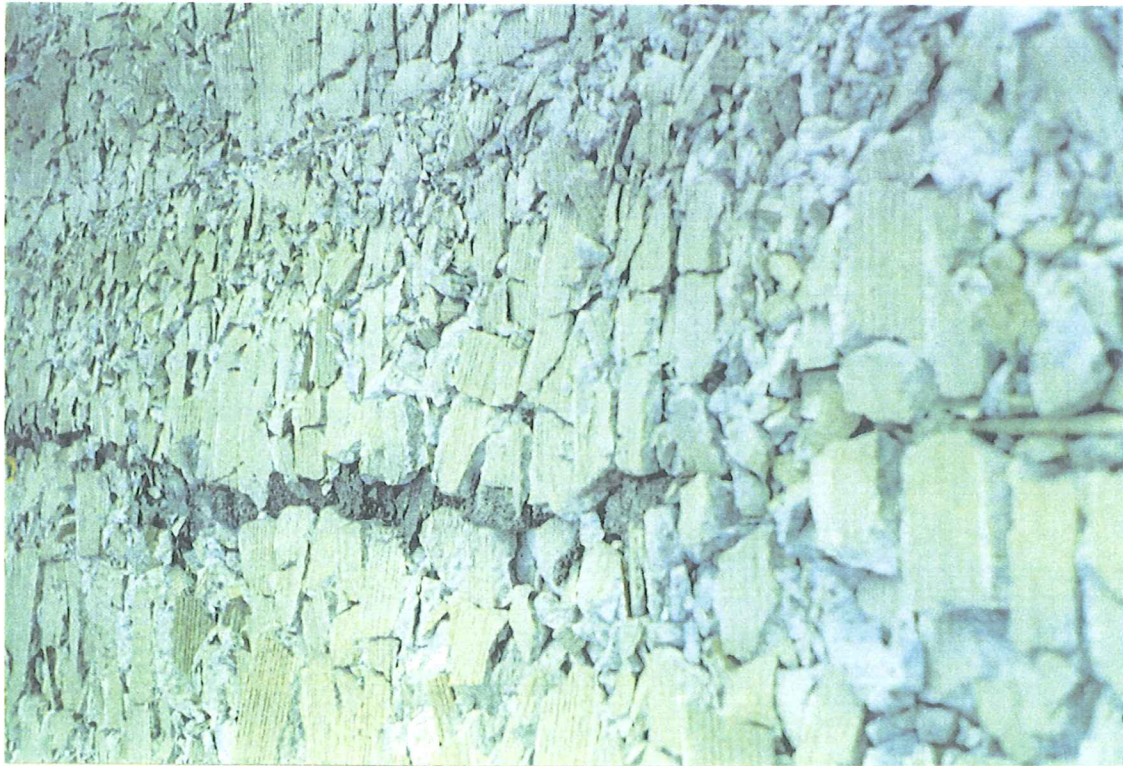
Showing how the CRC reinforcement bars followed the Longitudinal Cracks that had developed in the Concrete Pavement. The Picture on the left shows a crack filled with Bituminous Cold Patch prior to clean out to check location of the reinforcement bars
