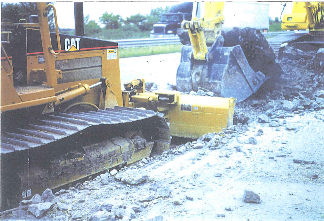
Showing pavement being removed by backhoe and OGDC and broken pieces of concrete being graded by bulldozer
