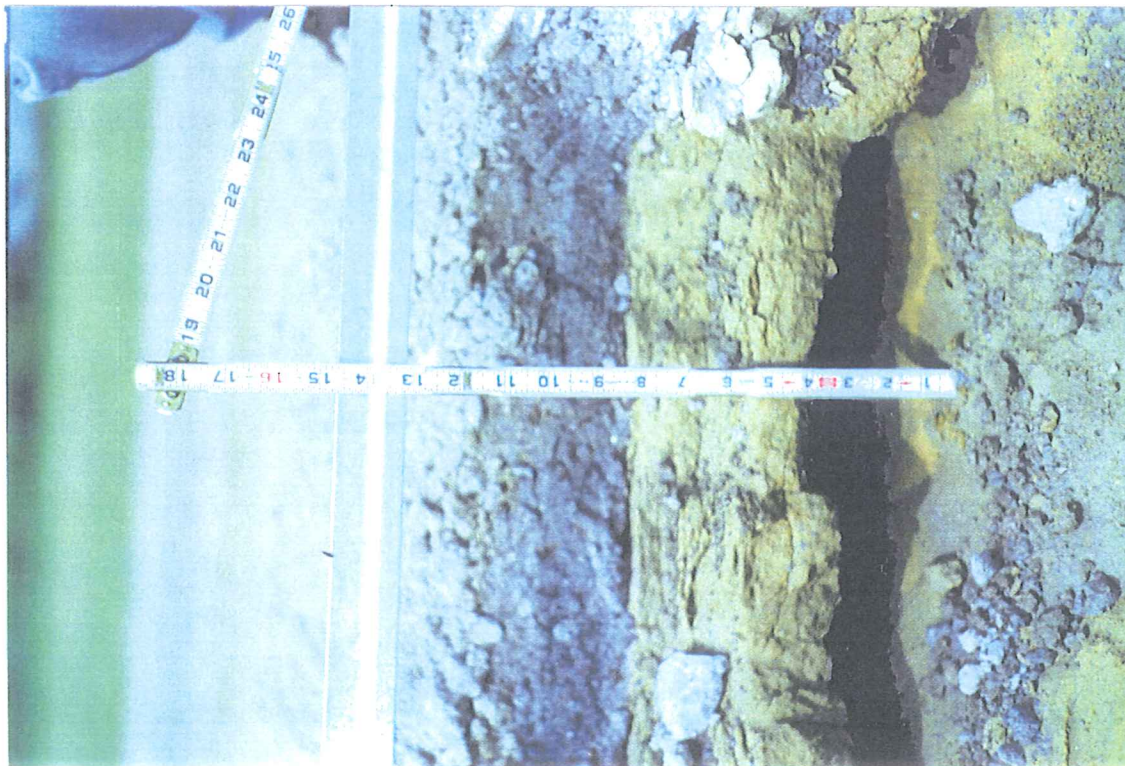
Showing Steel Furnace Slag used as Aggregate Base that had turned to a weak concrete and the sand subbase 4"-5" deep and an area where some of the sand subbase had washed out from under the sand subbase that had turned to a weak sand stone
