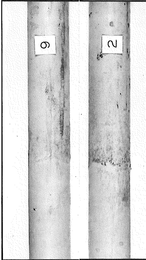
Figure 18. Plastic coated dowels after four years service show no corrosion.
