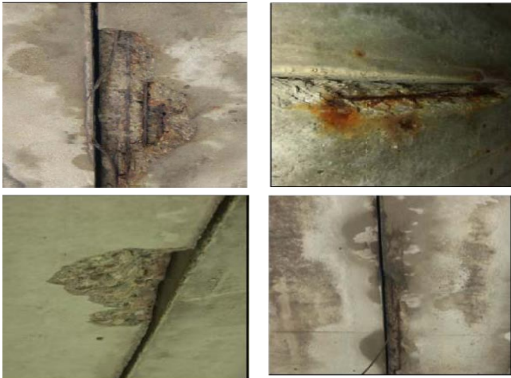
Figure 1.2-3 Deterioration of box beams at the shear key joints
