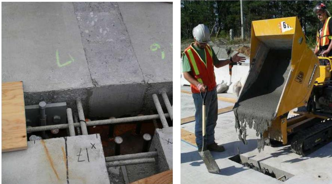
Figure 1.4-9 Joints ready for casting (left) and filling the joints with UHPC (right) in Rainy Lake Bridge, ON, Canada (Perry et al. 2009)
