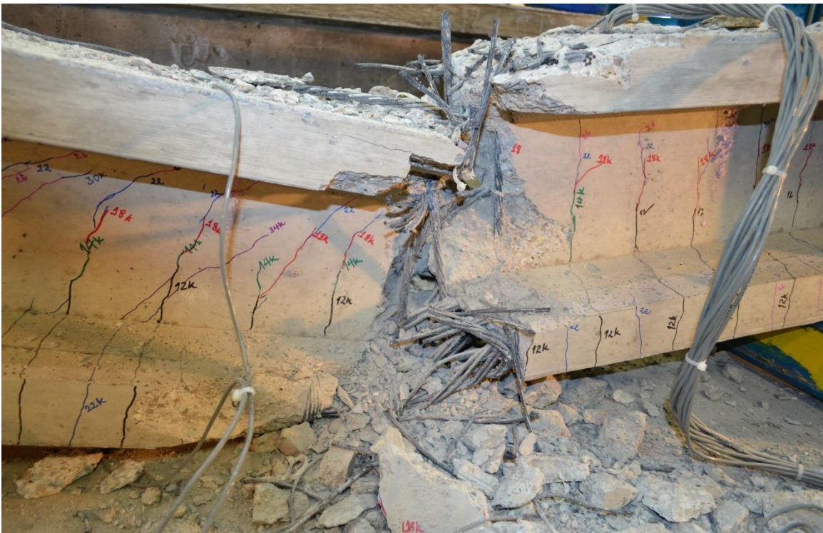
Figure 3.4-3 Close view showing the failure section of Beam C-S-F-O
