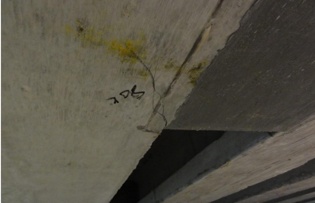
Figure 3.8-17 Cracks under a load of 80 kip near intermediate diaphragm
