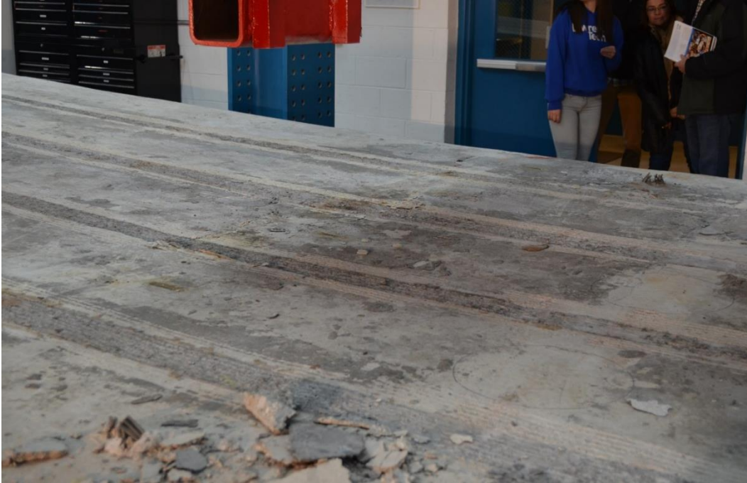
Figure 3.8-27 Partial concrete crushing in top flange after failure
