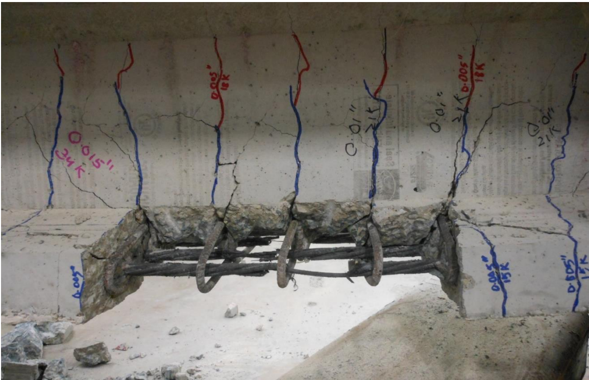
Figure 3.2-9 Rupture of prestressing CFCC strands in Beam C-S-F-U
