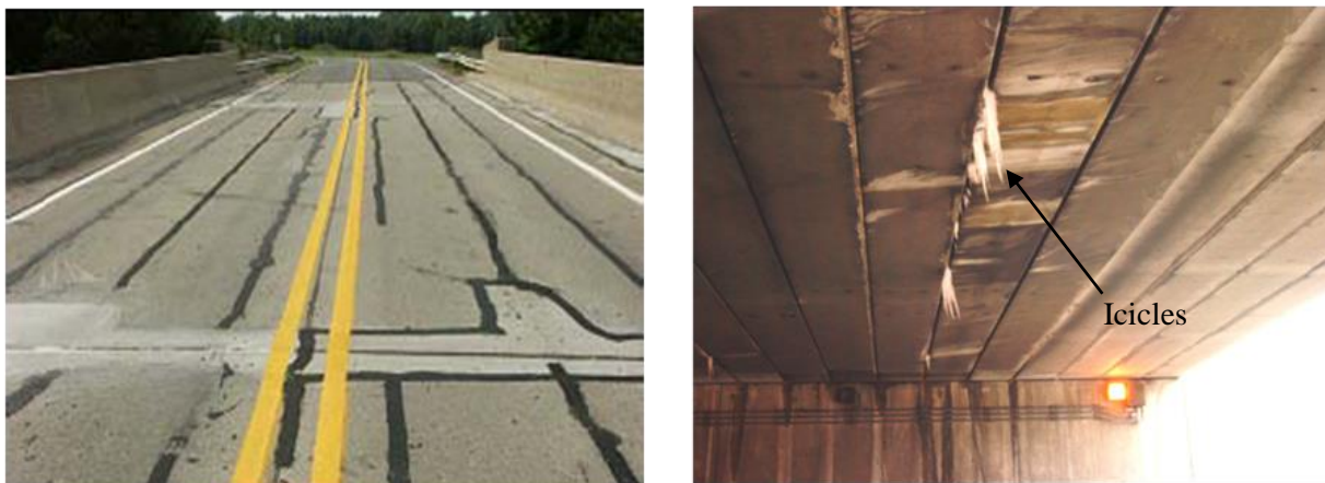
Figure 1.2-2 Crack development along the joints in side-by-side box beam bridges
