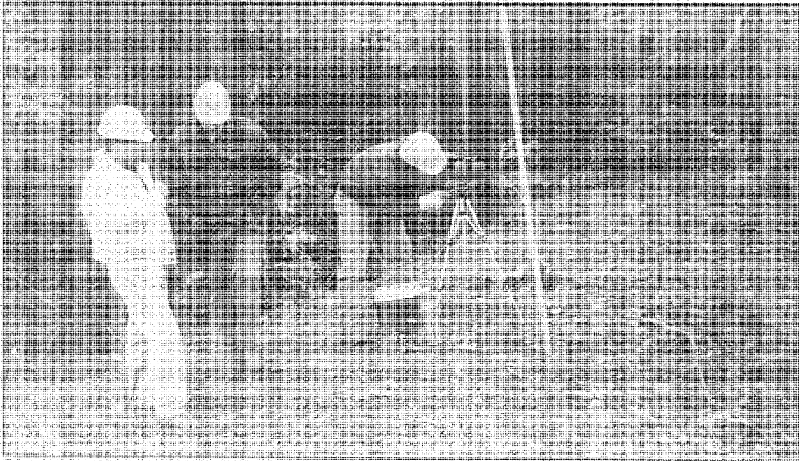
Figure 19: A Spotting Scope Was Used to Monitor Cracks in the Fascia Beams.
