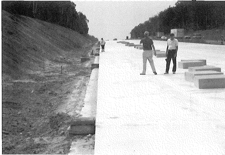
Figure 3.9 Construction site on the A10 south of Berlin showing catch basins at edge of slab that are connected to longitudinal pipe under the lean concrete base and connected to the manhole shown on the left.
