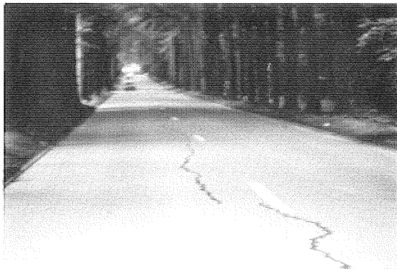
Figure 3.14 Dreve-de-Lorraine highway, Brussels, a 67-year-old jointed concrete pavement constructed in 1925 with no longitudinal joints.
