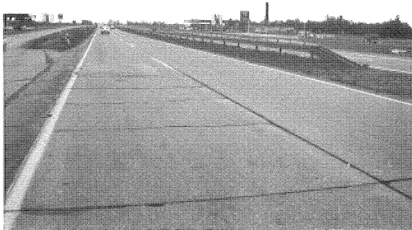
Figure 3.8 Photo of a 1930's German autobahn concrete pavement near Berlin. (Note cracking in outer truck lane of the 12-m (39-ft) slabs.)
