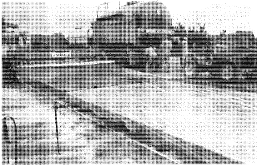
Figure 3.16 Polyethylene sheeting placed over concrete surface after retarder has been sprayed (Robuco process). (4)
