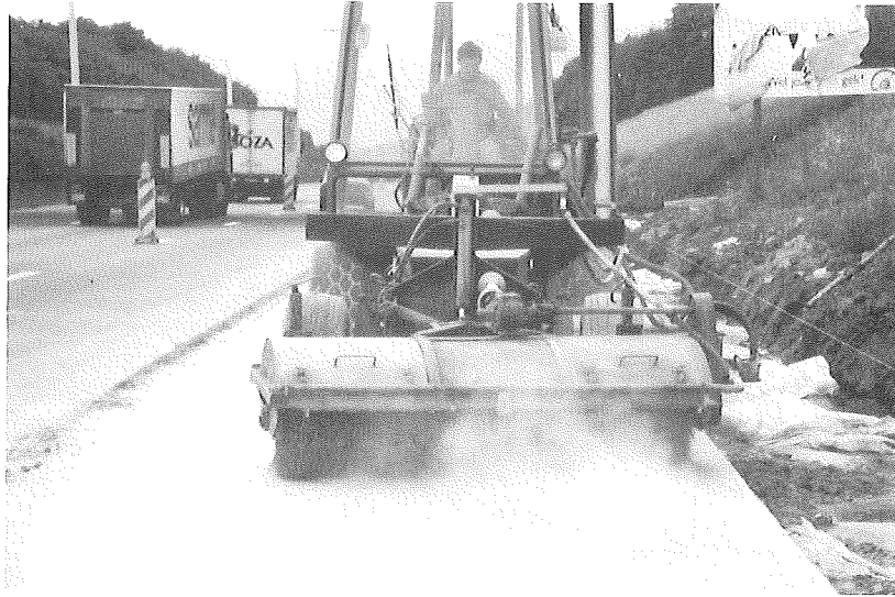
Figure 3.17 Rotary brush removing thin surface layer of mortar to provide the exposed aggregate surface after polyethylene sheeting has been removed.
