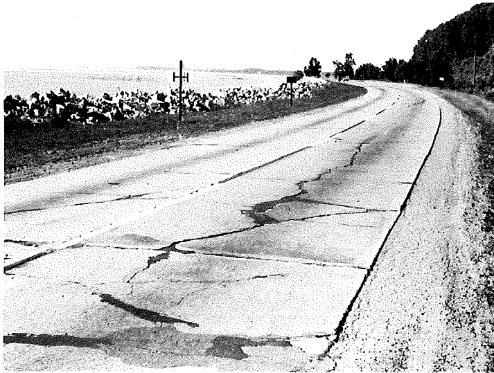
FIGURE 5. SECTION OF 21-6-C10 CONTAINING MANY TRANSVERSE CRACKS. 23 YEARS OLD.
