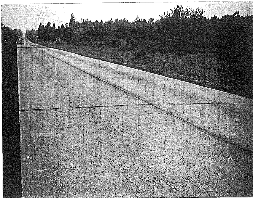
Figure 3. Project NRH 27-29, C2. Built in 1934. Champion fine and coarse aggregates, Beechwood. Surface shows little scale but has about two or three transverse cracks per 100-ft. slab. General view west from Sta. 447+00.
