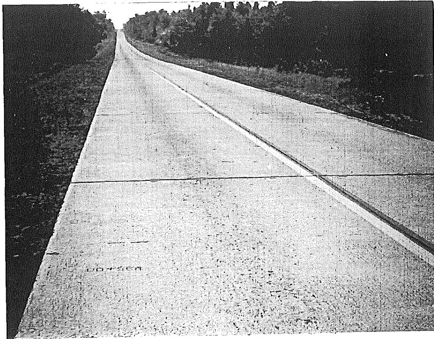
Figure 7. Looking west on Project 27-29, C4 from Sta. 896+00, showing general good condition of surface. Boniface aggregates.
