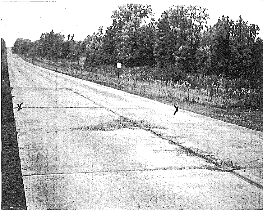
Figure 4. General view west showing junction of Project 27-29, C2 with Champion-Beechwood aggregates in background and 27-29, C4 with Boniface aggregates in foreground. Picture shows heavy scale at 622+50 on Project 27-29, C4.
