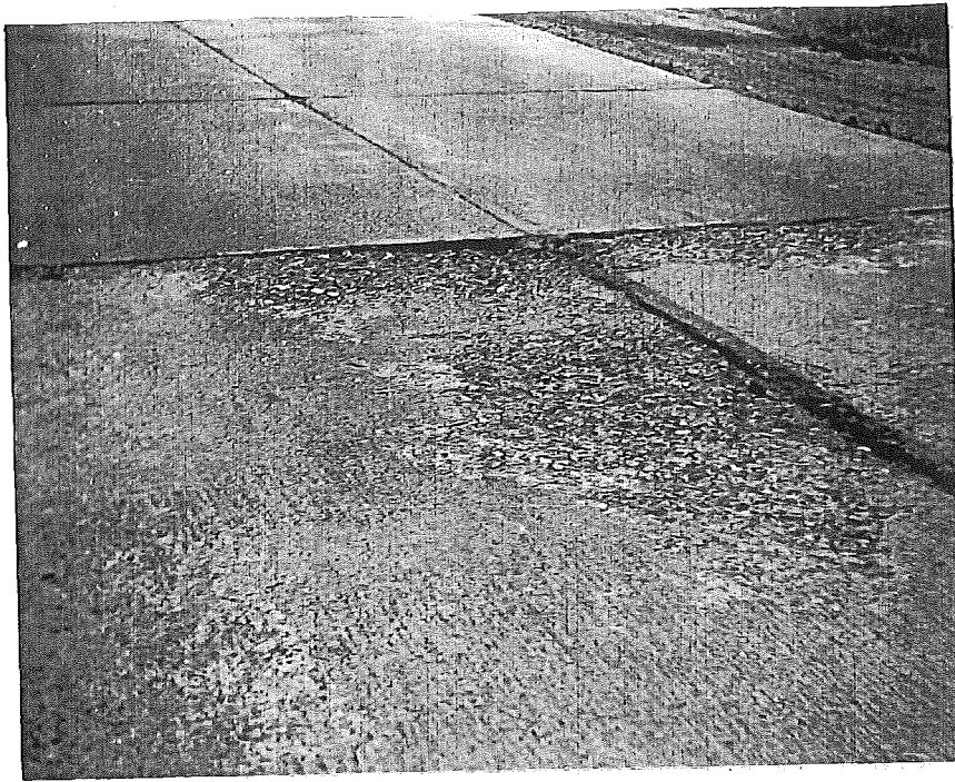
Figure 6. Joint to bridge approach at Little Presque Isle River, Sta. 697+74, Project 27-29, C4. Boniface aggregates and Petoskey cement. Bridge approach in foreground.
