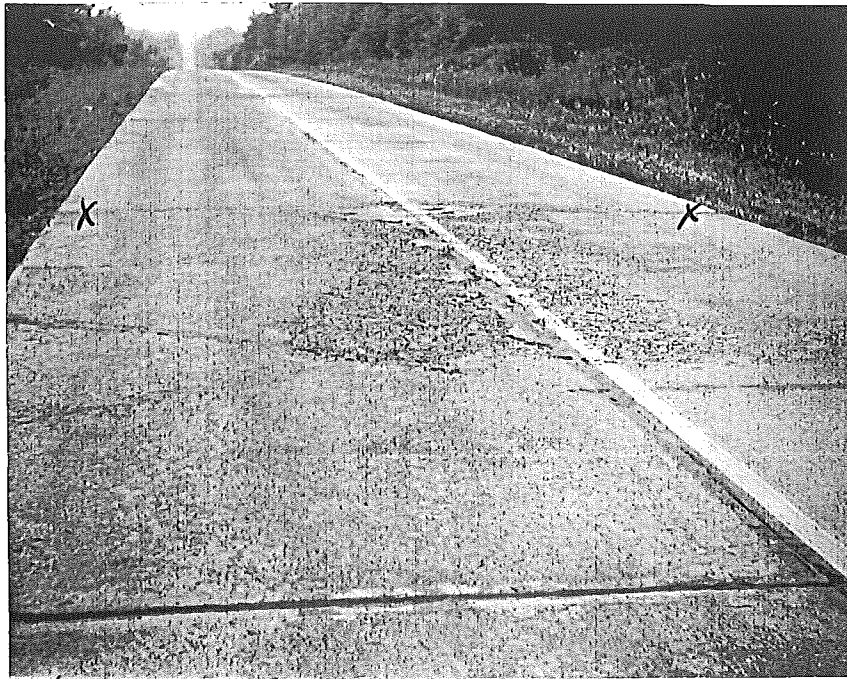
Figure 5. Construction joint between pours of 10-15-35 (foreground) and 7-31-36, Project 27-29, C4, Boniface aggregates. Note difference in condition of concrete on opposite sides of joint, Sta. 720+70. Same condition exists at other end of day's pour.
