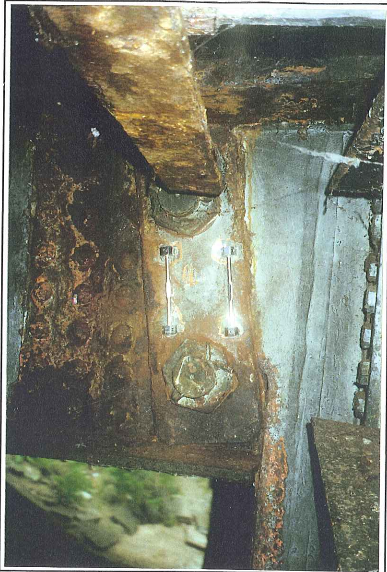
FIGURE 5 - Expansion joint has closed causing the beam ends to push against each other. (Structure Number B02 of 41027).
