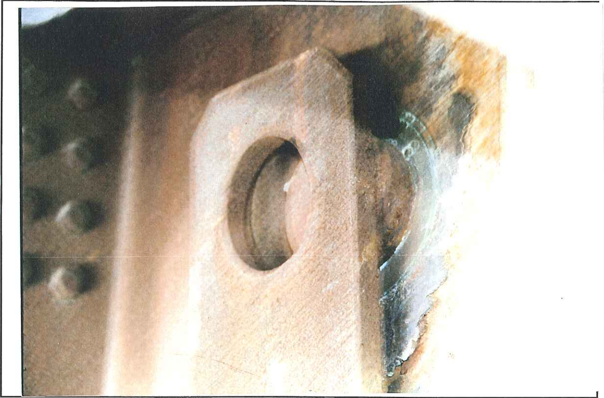
Figure 9. Link plate disengaged from pin. (Structure Number S15 of 82292)
