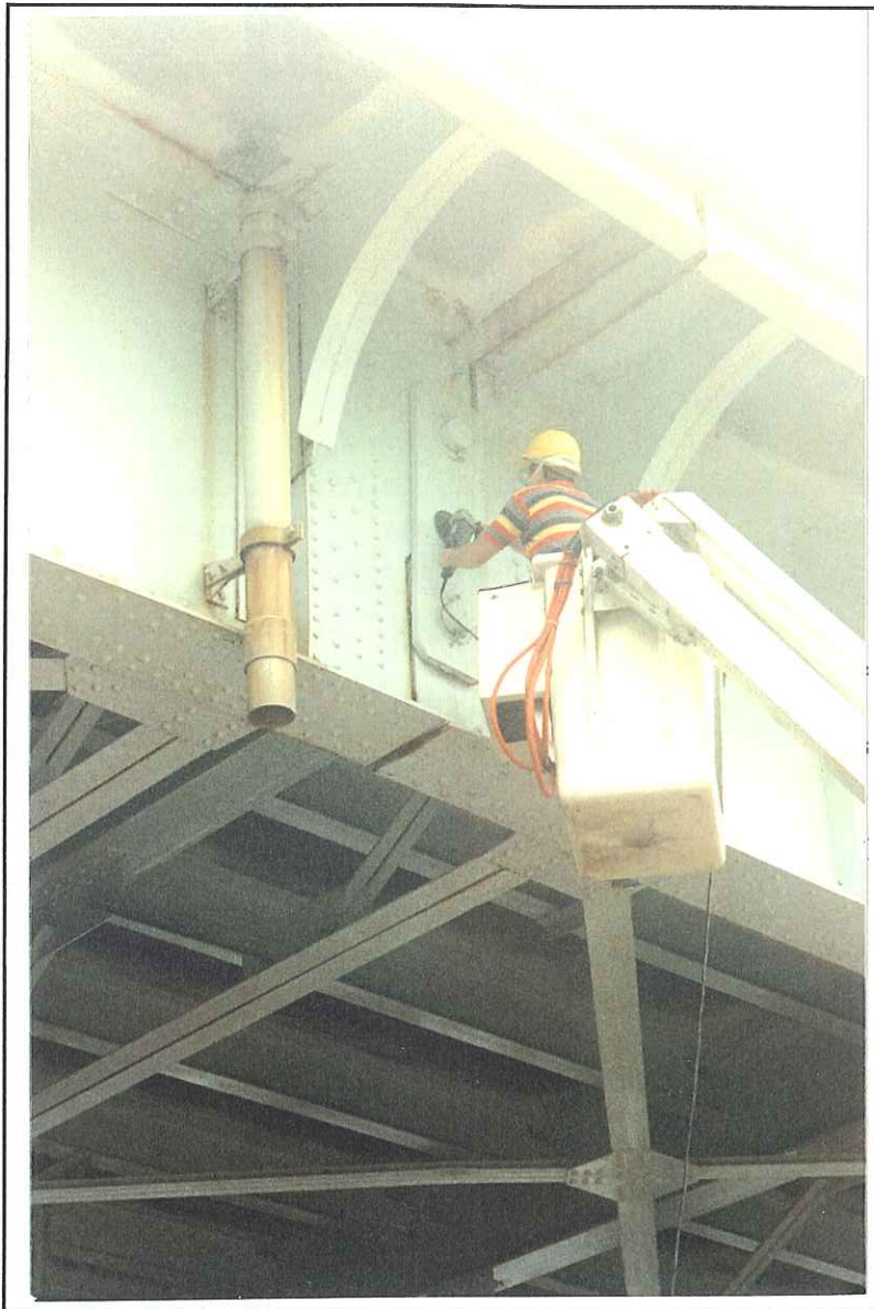
Figure 30. Link Plate. M-14/US-23 over the Huron River and Conrail Railroad. Note: Technician is preparing link plate for strain gage.
