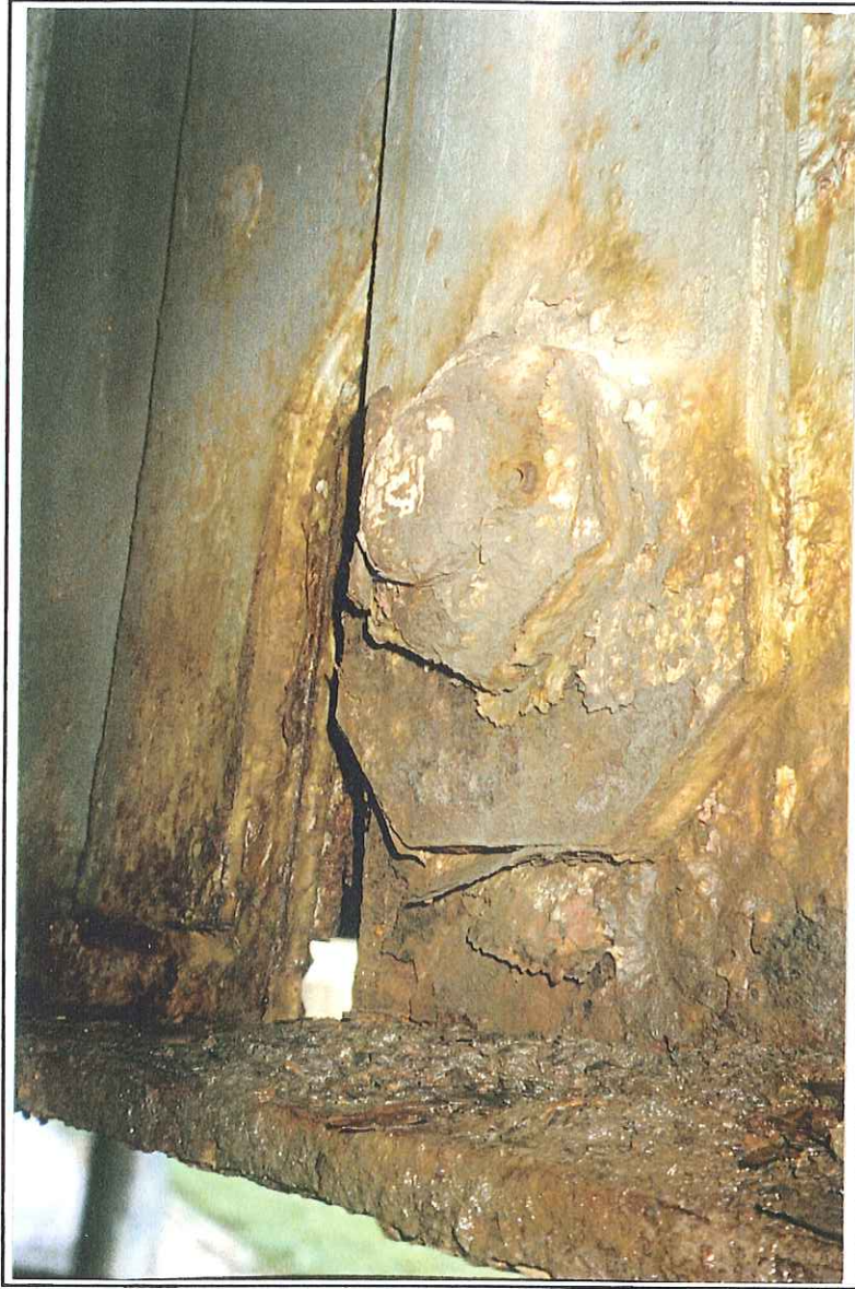
Figure 37 - Link Plate. I-75 over Toledo/Dix Highway.
