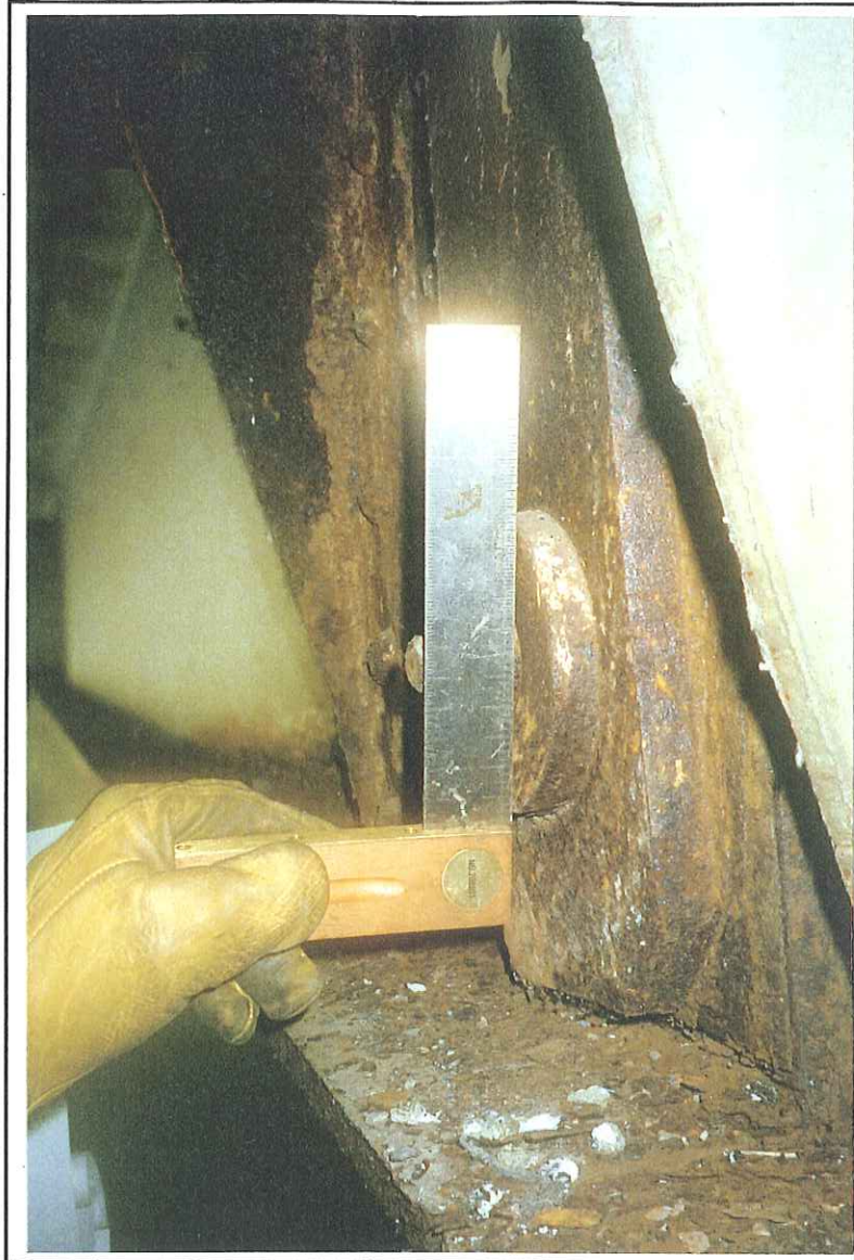
Figure 4. Structure Number - B04 of 58152. Corrosion build-up between the link plate and beam web is causing the link plate to move to the end of the pin, resulting in “cupping” of the pin cover plate.
