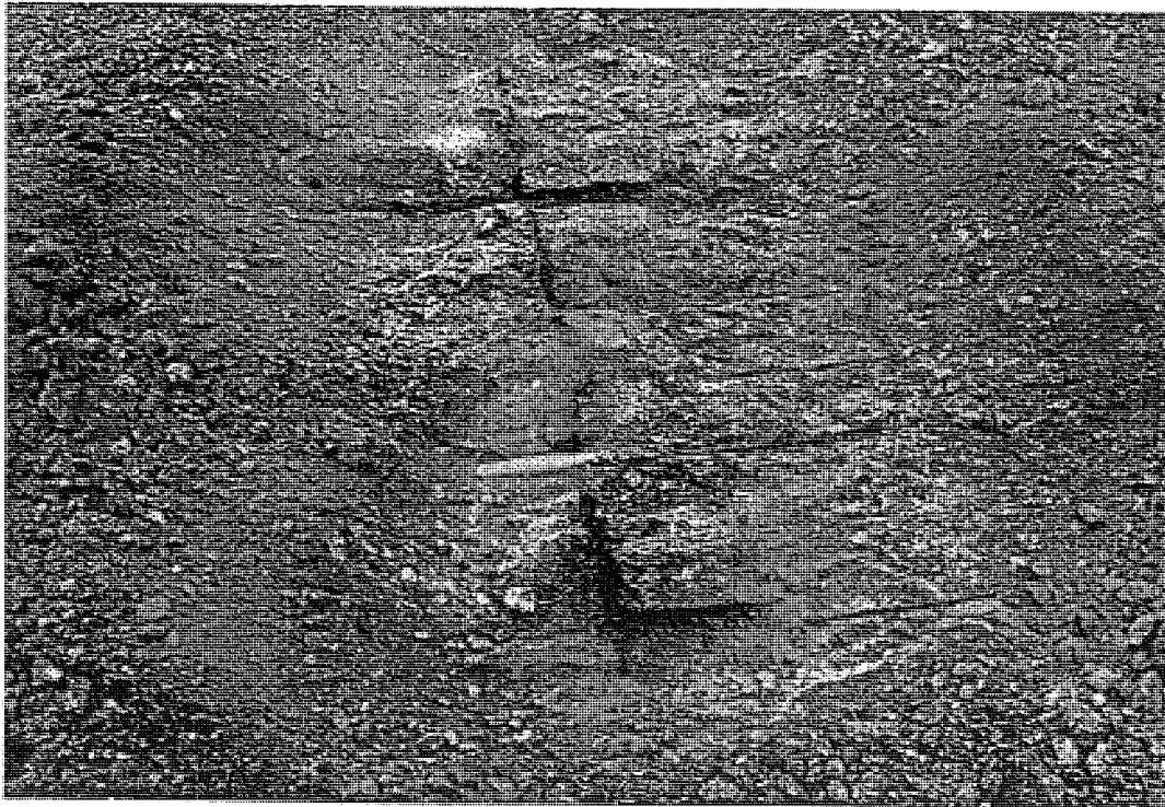
Figure 4.17 Partial destruction of the joint integrity (US-131)
