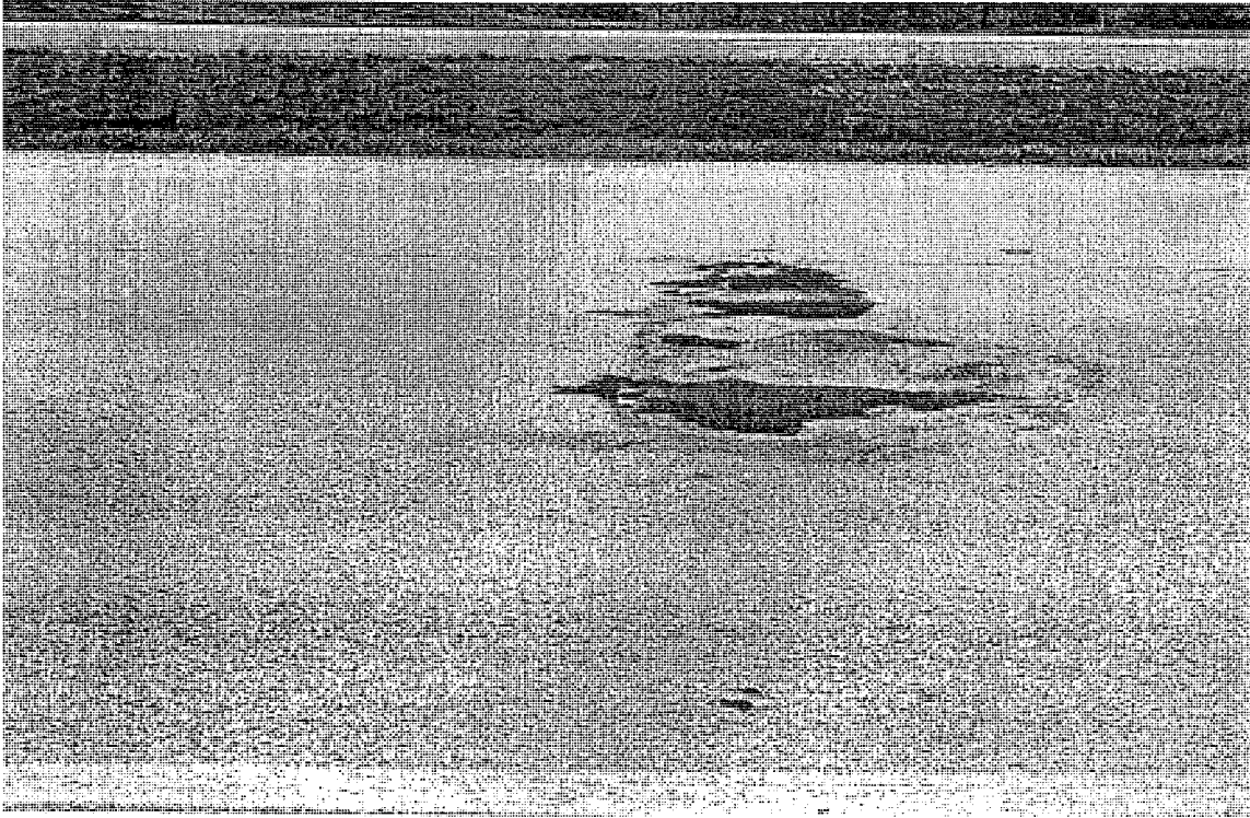
Figure 4.20 A shear failure along the rubblized pavement on NB I-196, May 2002
