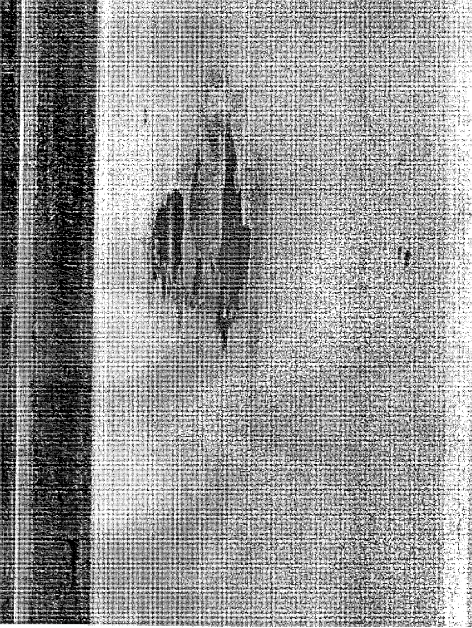
Figure 3.16 Shear failure along I-196 NB, Control Section 70024 Job Number 35987 BMP 12.6, EMP 15.6
