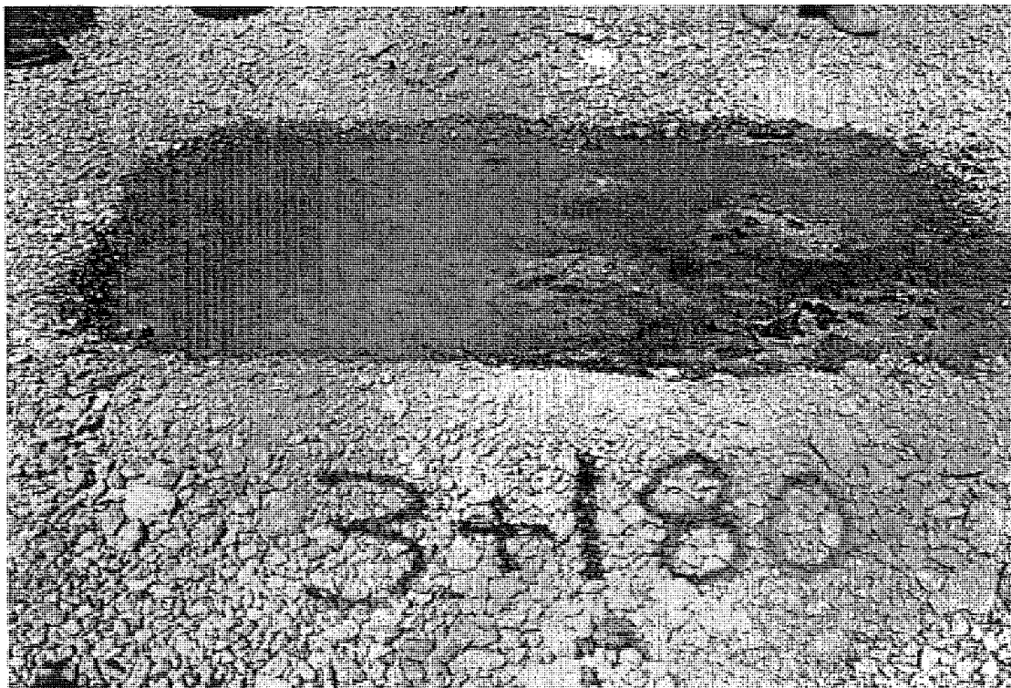
Figure 4.18 Trapped water above the fractured concrete in a trench along M-18
