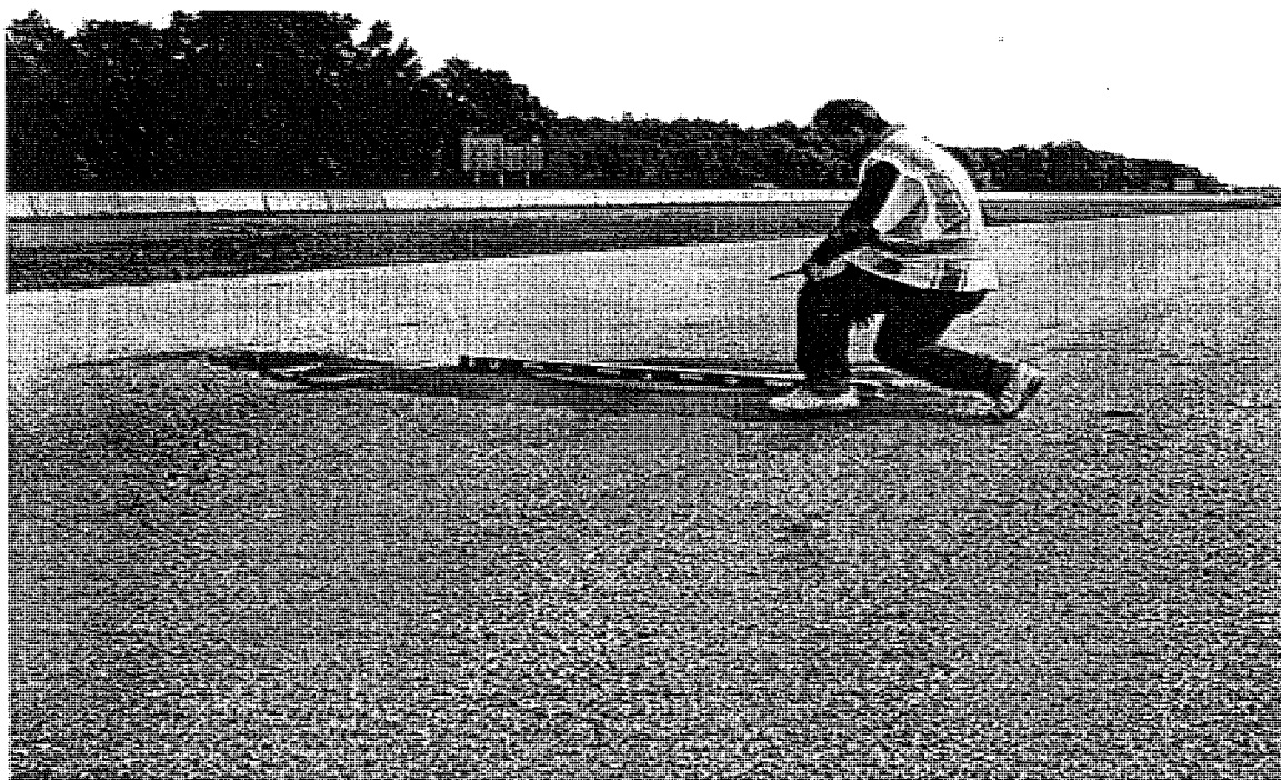
Figure 4.19 Shear failures in the rubblized pavement along NB I-196, August 2001
