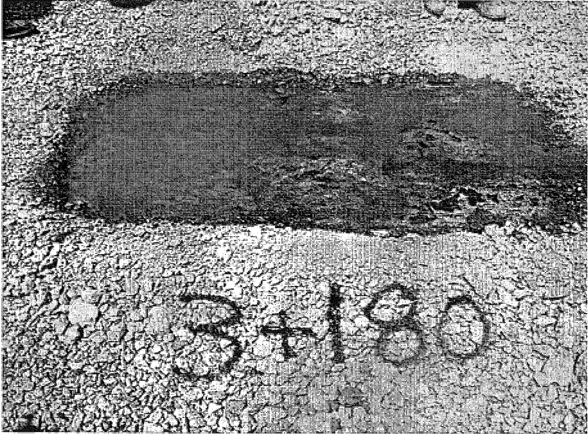
Figure 3.5 Trapped water above the fractured concrete in a trench (M-18)
