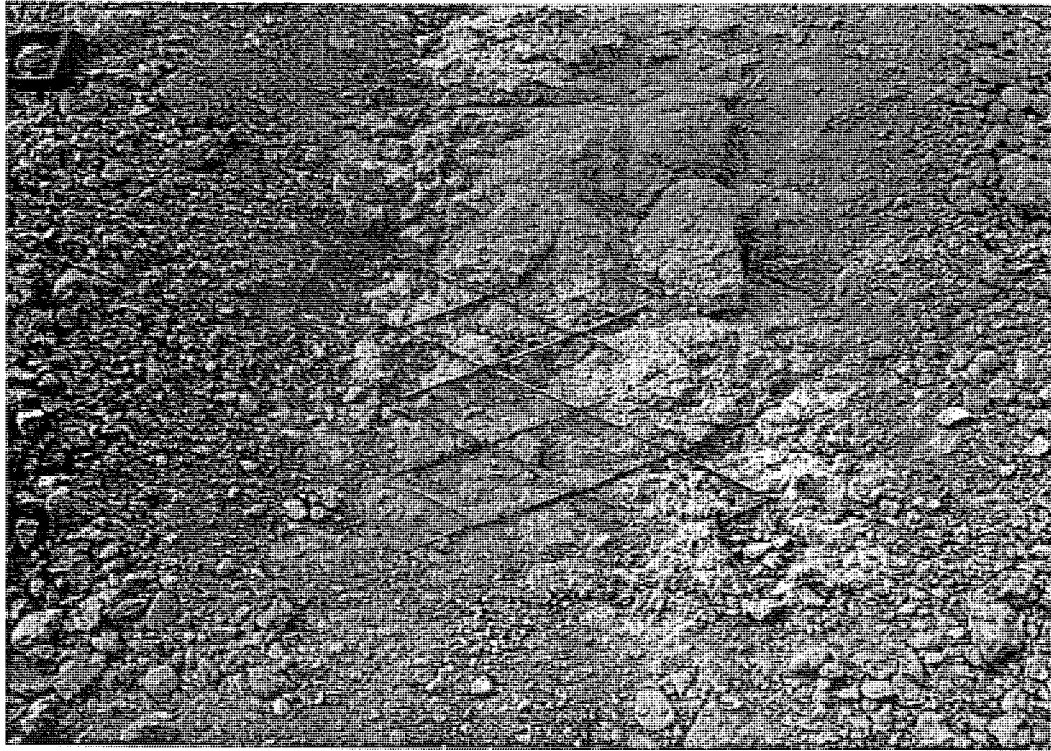
Figure 3.3 Partial debonding of the temperature steel (M21)
